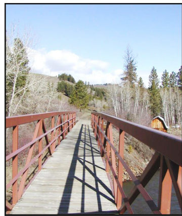
The Combs Trestle near Fruitvale offers a scenic crossing of the Weiser River. - Mary Ellen Pugh Photo
