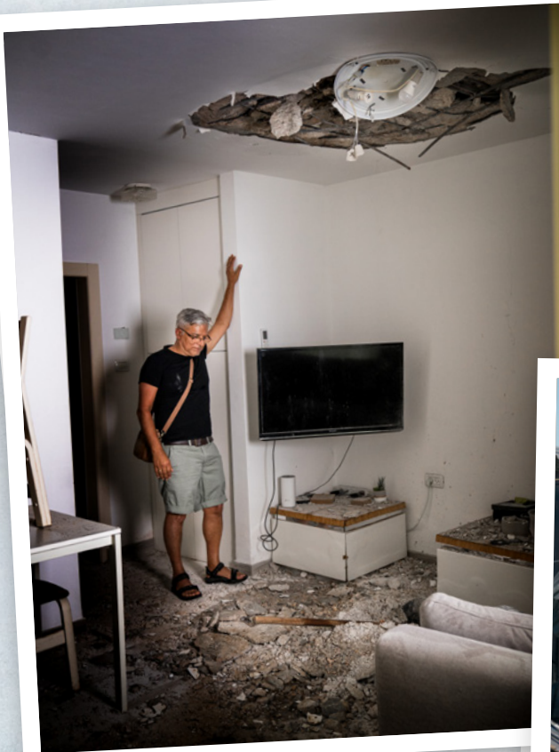
Hezi stands in what remains of his living room Right: View of destruction from the outside
