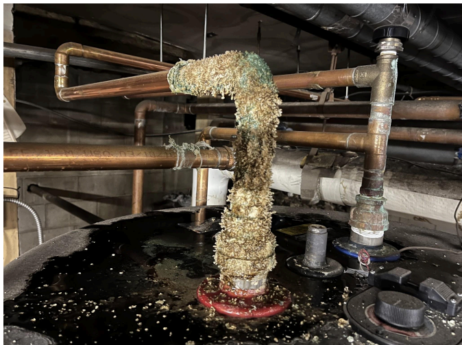
Top of another tank with corrosion and leaks
