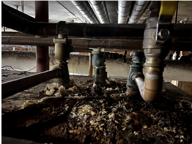
Top of one tank with corrosion from leaks.
