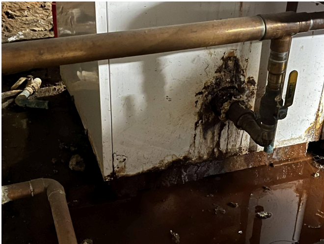
Supply water feed to tank inlet with corrosion and rust.
