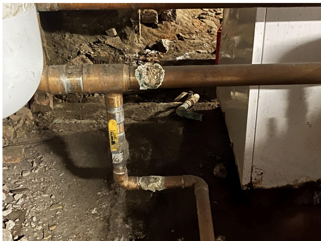
Supply water feed to tank inlet with corrosion from leaks.
