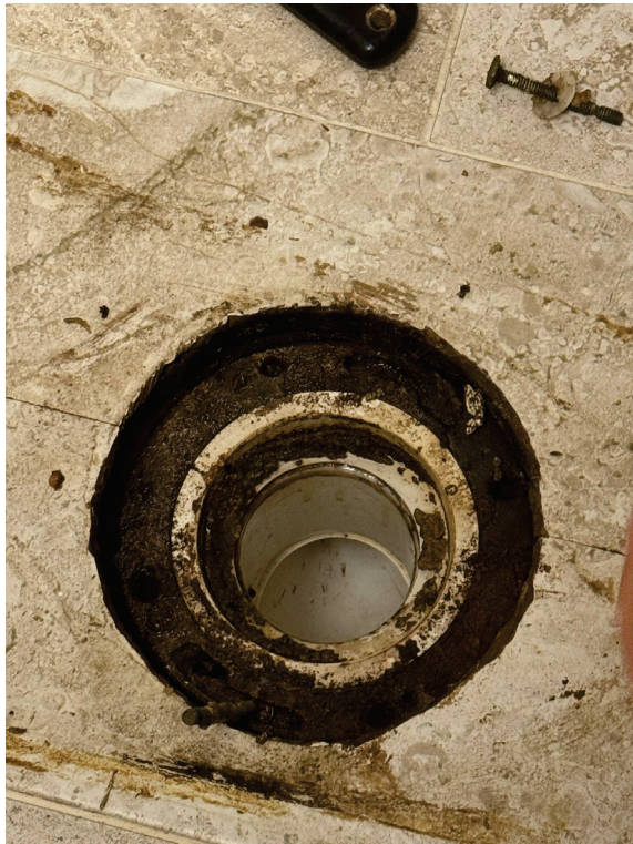
The toilet flange is approximately \frac{3}{4} of an inch below the floor surface.
