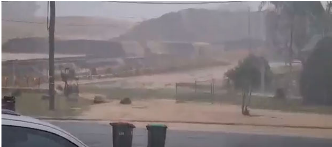
Storm water run off from Ridgeviews development site, July 2022
