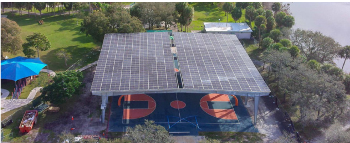
Two large-scale solar canopies over the basketball courts at Reverend Samuel Delevoe Memorial Park in Fort Lauderdale.
