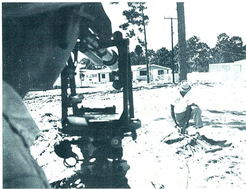
SIGHTING ON THE SITE —Surveying crew takes final sighting to determine exact location of Imperial Point home. Purchaser has previously selected desired lot. Following report of survey, building crews will move in to commence job.
