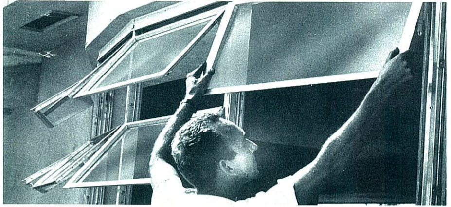
ALUMINUM AWNING WINDOWS GO INTO PLACE —Installation man places awning windows in already mounted aluminum framing. Each pane of glass is framed in heavy-duty aluminum and weatherstripped for weathertight closure. Awning windows provide maximum ventilation and may be safely left open during rain.
