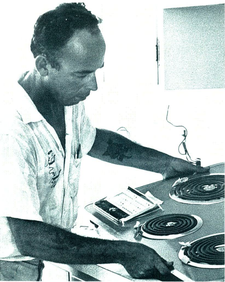
← GETTING THE RANGE —General Electric installation man sets counter top electric range in place in mica kitchen counter. GE wall oven (not shown) has already been installed.
