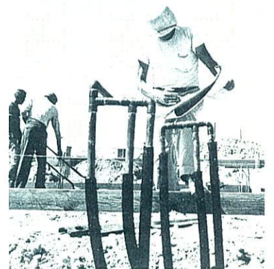
LAST CHECK BEFORE POURING FOUNDATION SLAB — Haft-Gaines foreman, blueprint in hand, makes final detailed check of preparatory work on site. When his O.K. is initialed on plans, foundation slab will be poured and home will be off to a proper start.
