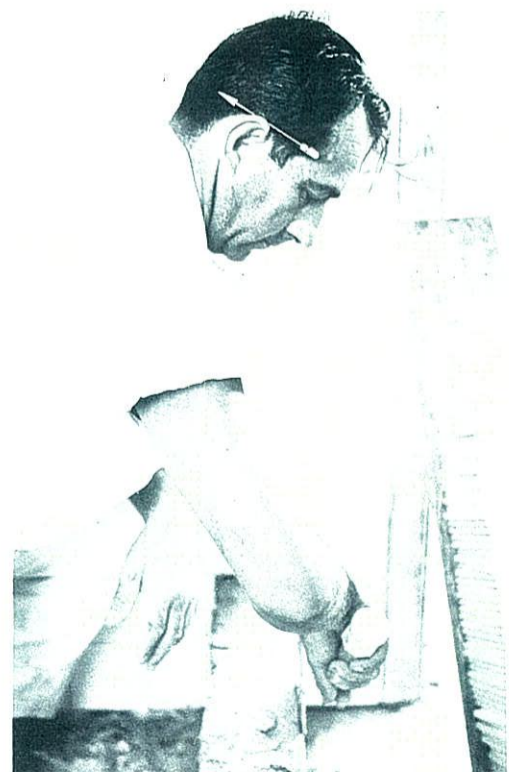
SETTING TILES —Bathroom ceramic tiles are installed following placing of bathroom fixtures. Colors are chosen by purchaser from a wide variety before construction begins.
