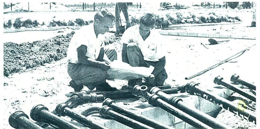
NO PIPE DREAM — Pipe counter and pipe checker check line-up of pipe against blueprints to make sure every specified item is accounted for. Pipe will be set in foundation form preparatory to pouring slab.
