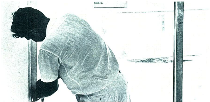
SLIDING GLASS DOORS —Smoothly rolling glass doors set in aluminum frames open onto patios. Crews check locking, weather-stripping, fingertip action before approving installation.
