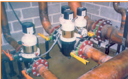
Drinking water filtration using JPF-ATP DN 100 and DN 150 Olympic village Sydney, Australia
