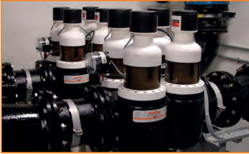
Drinking water filtration using JPF-ATP DN 200 City of Dreams Casino Resort Macao, China
