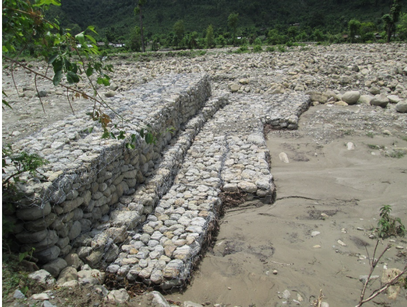
Figure 31. Gabions installed to help prevent additional erosion where gravel excavation has taken place.
