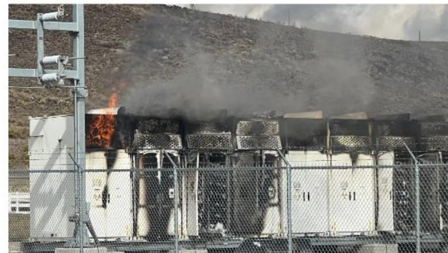
Idaho Power substation battery fire (courtesy Canyon County Sheriff's Office)
