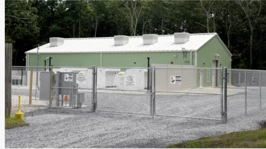
The 5-megawatt battery storage unit, located in East Hampton, has been out of service since a fire in May. Credit: Veronique Louis
