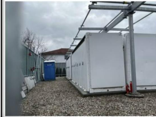
Very energy storage site at Littlefield Avenue and Hylan Boulevard in Littlefield is pictured here. Fires at two battery energy storage sites in Warwick, N.Y., have been smoldering for more than a week, after officials say a common-related issue caused the newly installed units to ignite and burn in two separate incidents last month. (Staten Island Advance/Jan Somma-Hammel)
