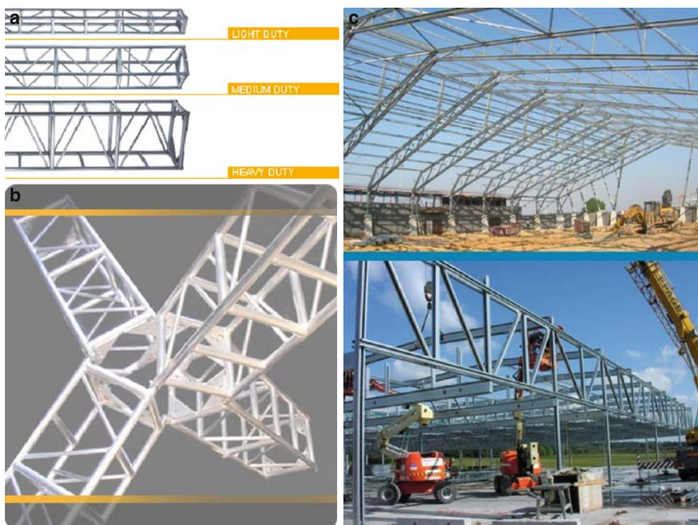
Fig. 5.9 Examples of architectural trusses. (a) and (b) From TotalStructures.com. (c) Example of articulated architectural trusses in building. (voestalpine.com)
