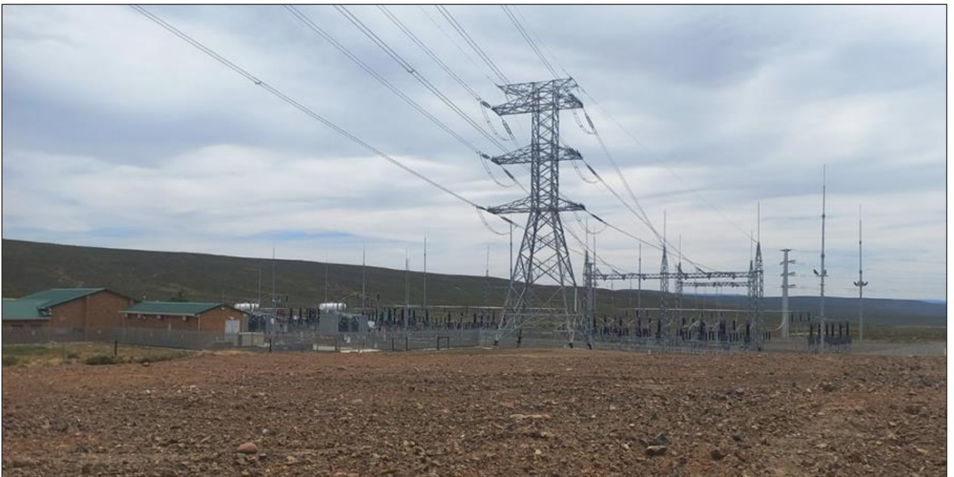
Figure 4: Ripping completed at tower foundation (Bon Espirange Substation) (photograph courtesy of Mahle Myaka)
