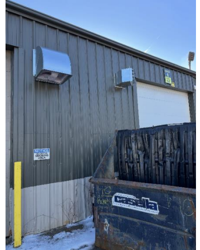
Outdoor exhaust and intake vents.
