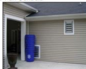
Fig. 3 – Exhaust and Intake louvres for ERV
