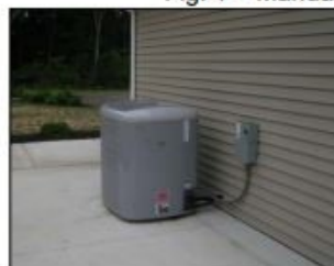
Fig. 2 – High-Efficiency Carrier split system
