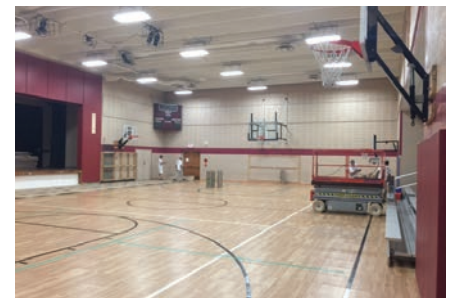
▲ Working around wiring and lights added to the challenge of the ceiling painting.
