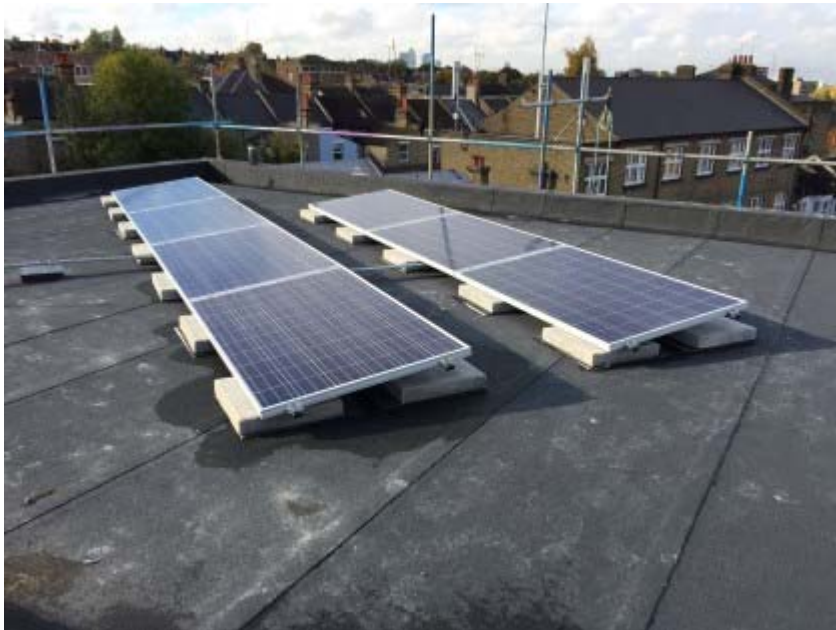
Photo 6: Typical flat roof mounted ballast system
