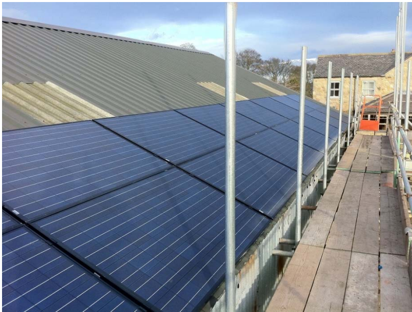
Photo 4: PV panels being installed on a barn roof (photo courtesy of Geowarmth)
