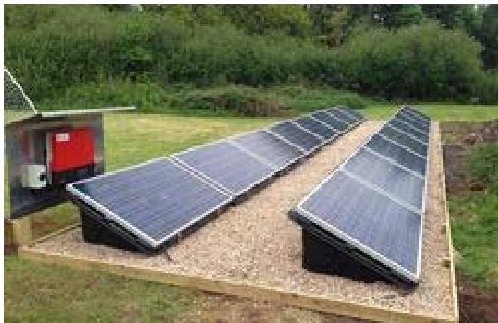
Photo 7: Ground mounted ballast system
