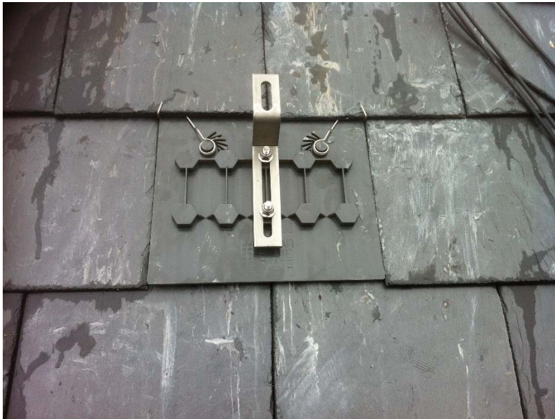
Photo 13: A simple solar installation on slate roofs by solarslateplate.co.uk
