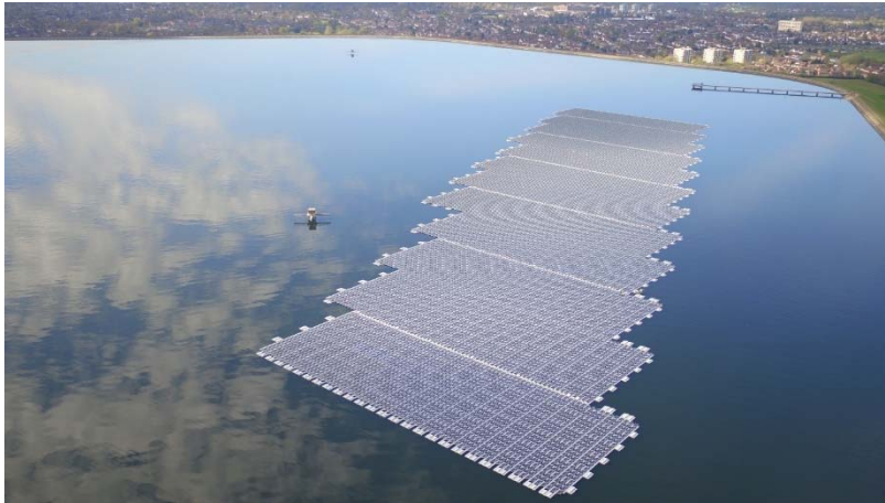
Photo 8: The Lightsource bp 6.4MW floating PV array on London's Queen Elisabeth II reservoir
