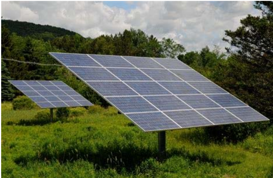
Photo 11: Pole mounted tracking PV
