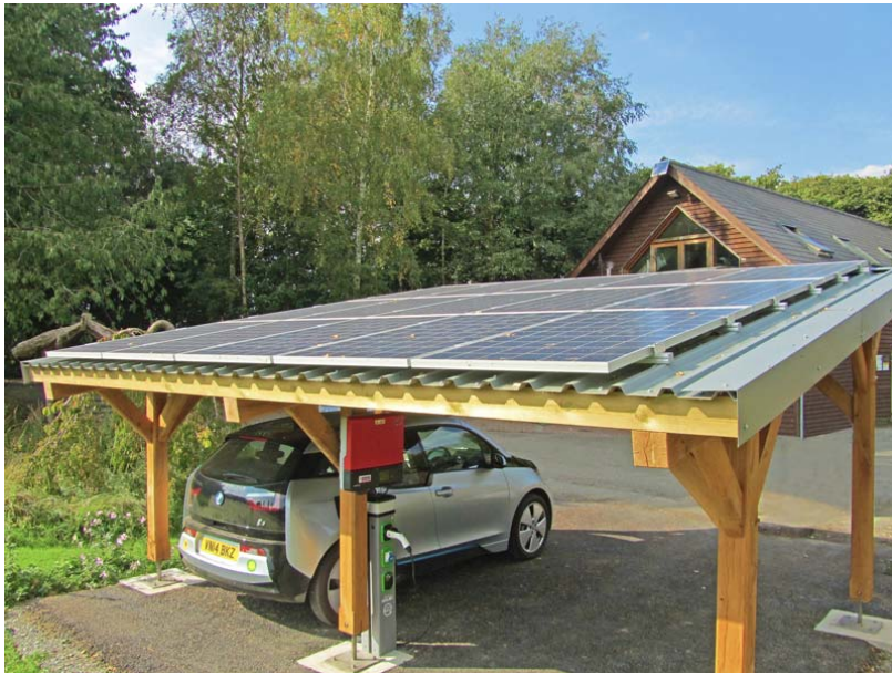
Photo 9: Solar PV car port
