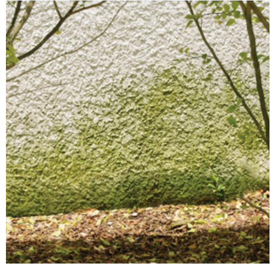
Picture 1: Before NeverFade was installed — mold and algae growth on shaded areas of the facade.
