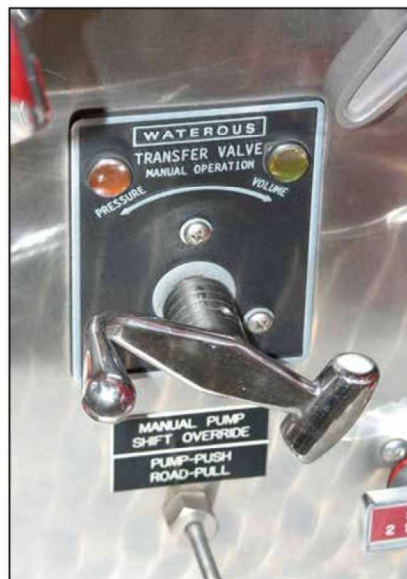
Figure 9.9 Pump operators use a transfer valve to switch between volume and pressure pumping operations.
