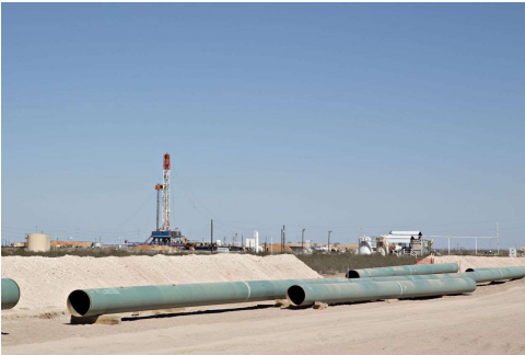
Bottlenecks have become a problem in the Permian Basin of Texas and New Mexico at the center of the shale boom. Sections of pipeline lay on the ground near an oil drill rig near Pyote, Texas, on March 2. PHOTO: DANIEL ACKER/BLOOMBERG NEWS
