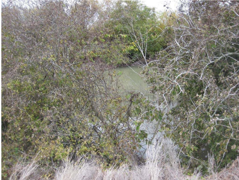
Photo 76 –Drainage feature at Plot PL-22
