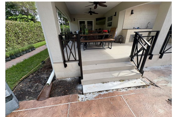
Entry step rail
