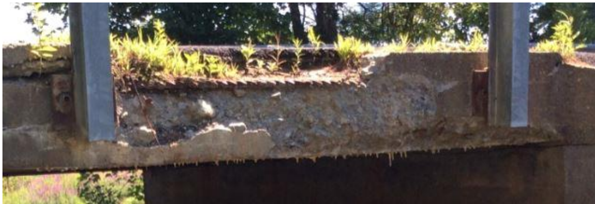
An example of severe concrete spalling.
