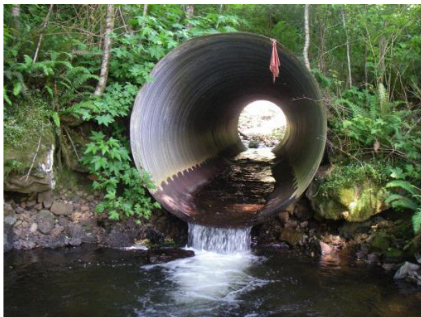
The outlet of this metal pipe is perched 2 feet above the downstream water surface, so is classified as a free fall.
