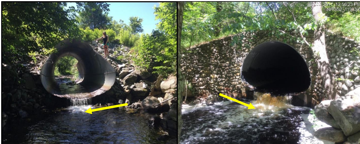
The water depth is measured right at the point where water spills into the stream from the outlet.
