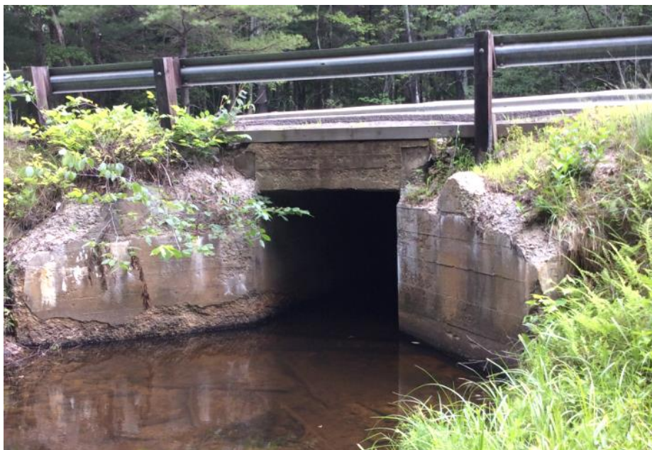
Box culvert with poor inlet condition due to significant spalling, cracks in concrete, and loose stones.
