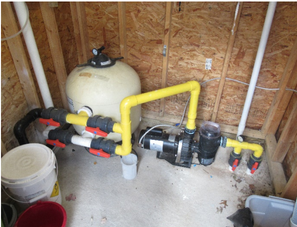
Pump and filter overview, wading pool
