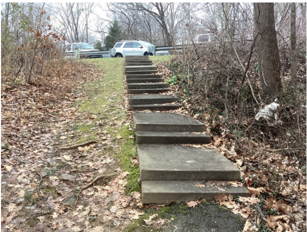
Concrete stairs overview, North trail (Note: Uneven steps and landings.)
