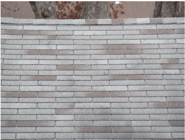
Asphalt shingle deterioration and staining, wading pool shed
