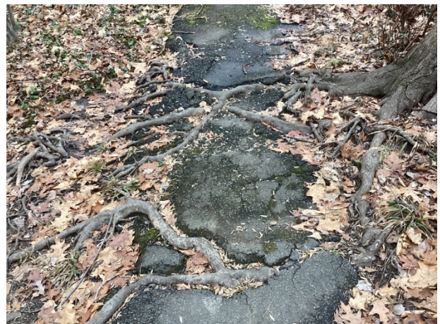
Asphalt crack and tree root damage
