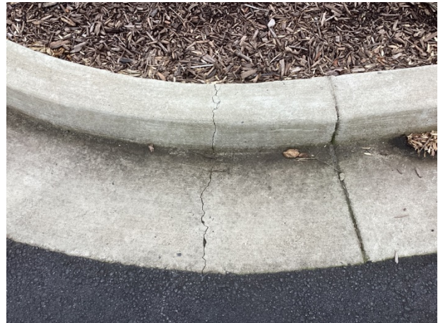
Concrete curb and gutter crack
