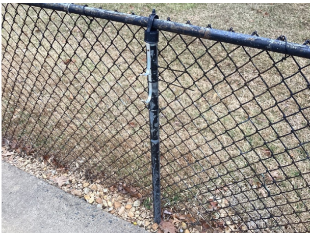
Finish deterioration at wading pool fence
