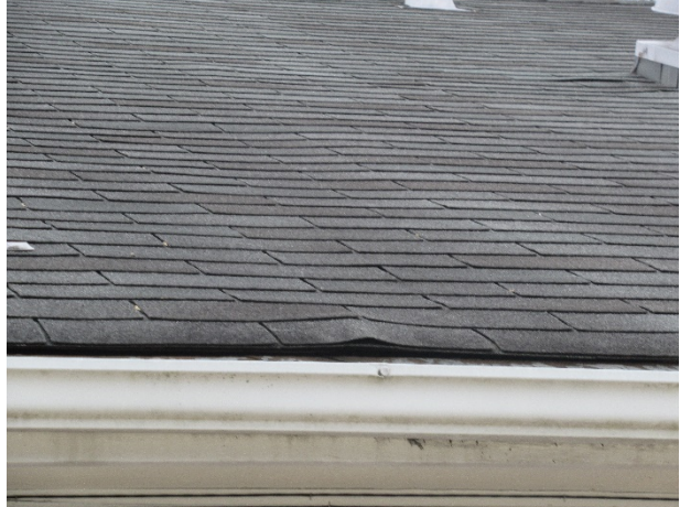
Asphalt shingle lift
