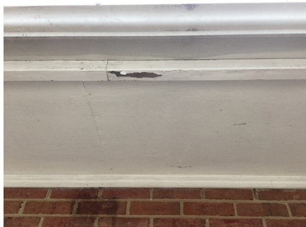
Soffit finish deterioration overview
