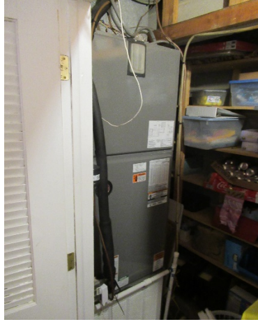
Air handling unit overview
