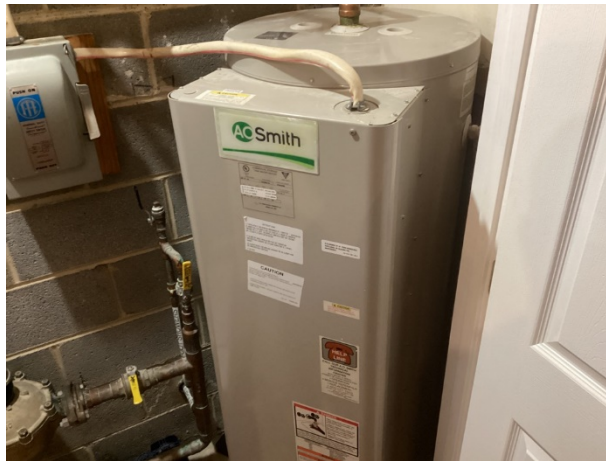
Water heater overview
