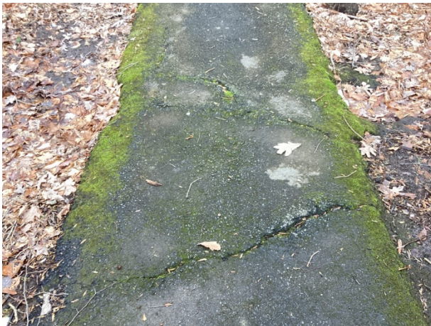
Asphalt cracks and organic growth
