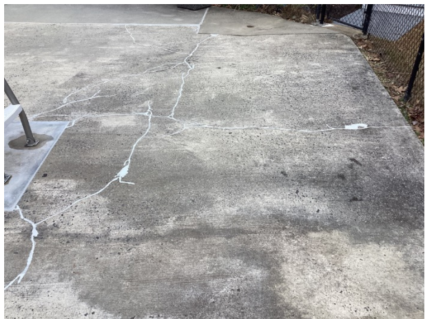
Concrete deck previous repairs and staining
