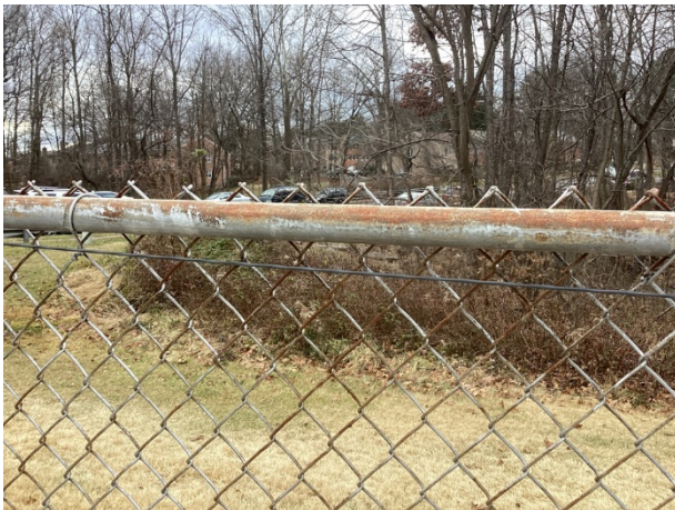
Rust at security chain link fence
