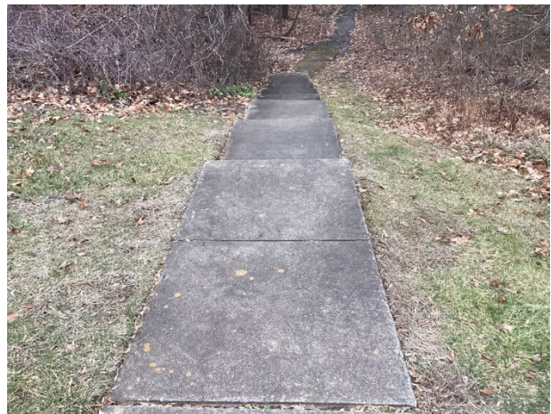
Concrete stairs overview, South trail, #1 (Note: General concrete deterioration and staining.)
