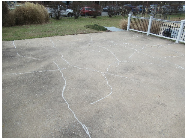
Concrete deck previous repairs
