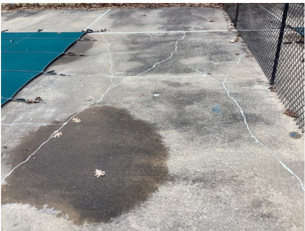
Concrete deck previous repairs and staining
