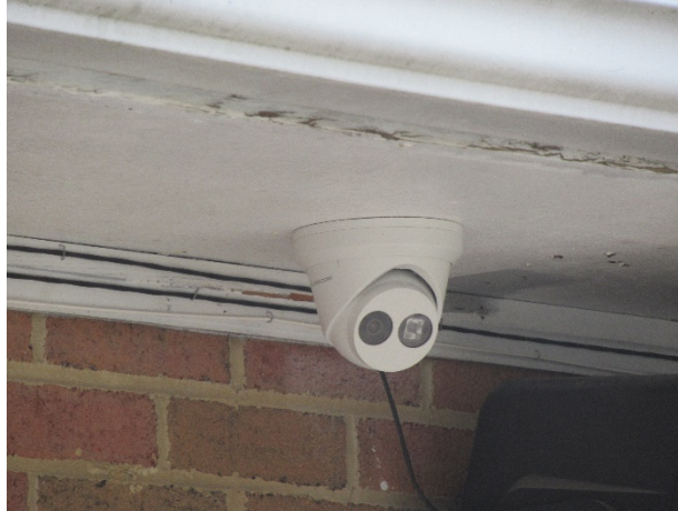
Security camera overview
