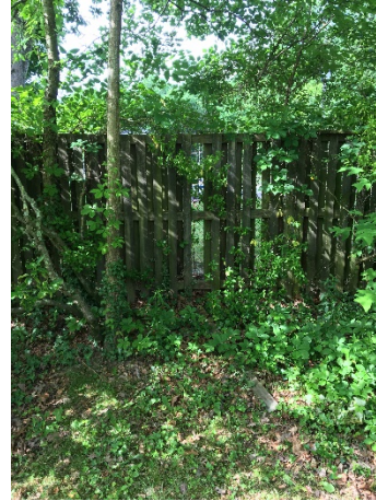
Overgrown section (Note: this image was provided by the Association)
