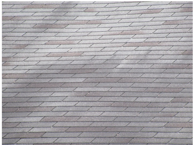
Asphalt shingle deterioration and staining, storage shed
