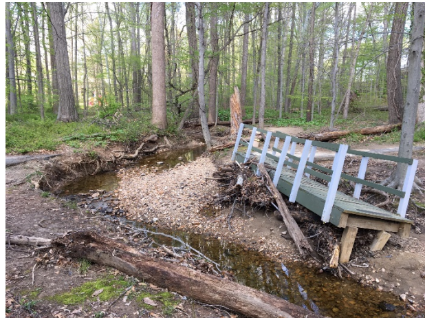
Damaged bridge connecting South trail and Kara trail
