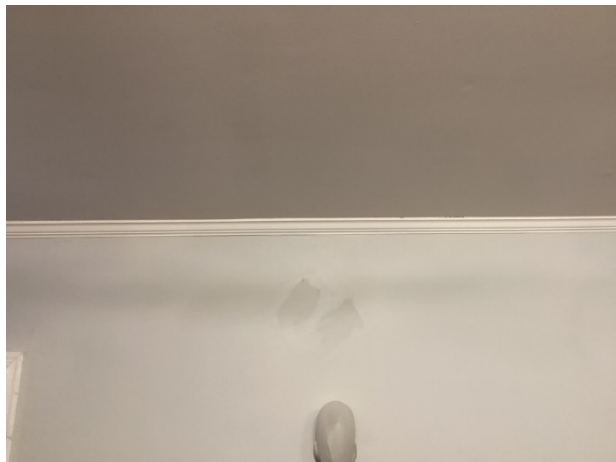
Finish deterioration at the walls
