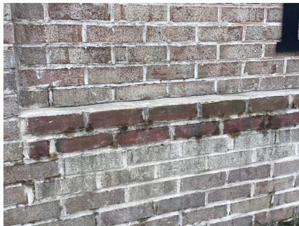
Brick masonry efflorescence and deterioration
