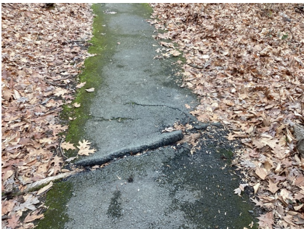
Asphalt crack and tree root damage
