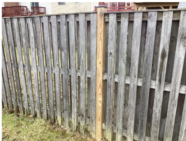
Wood perimeter fence overview (Note: Previously repaired post.)
