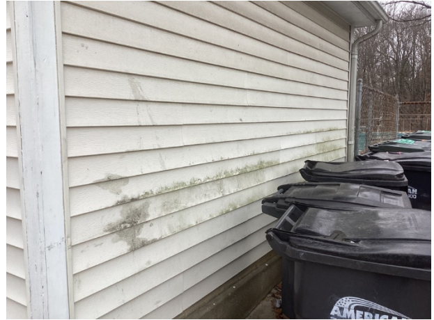
Staining at the sheds
