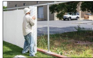
Fence installer installing a roll of chain link fence with factory inserted slats already in the wire.
