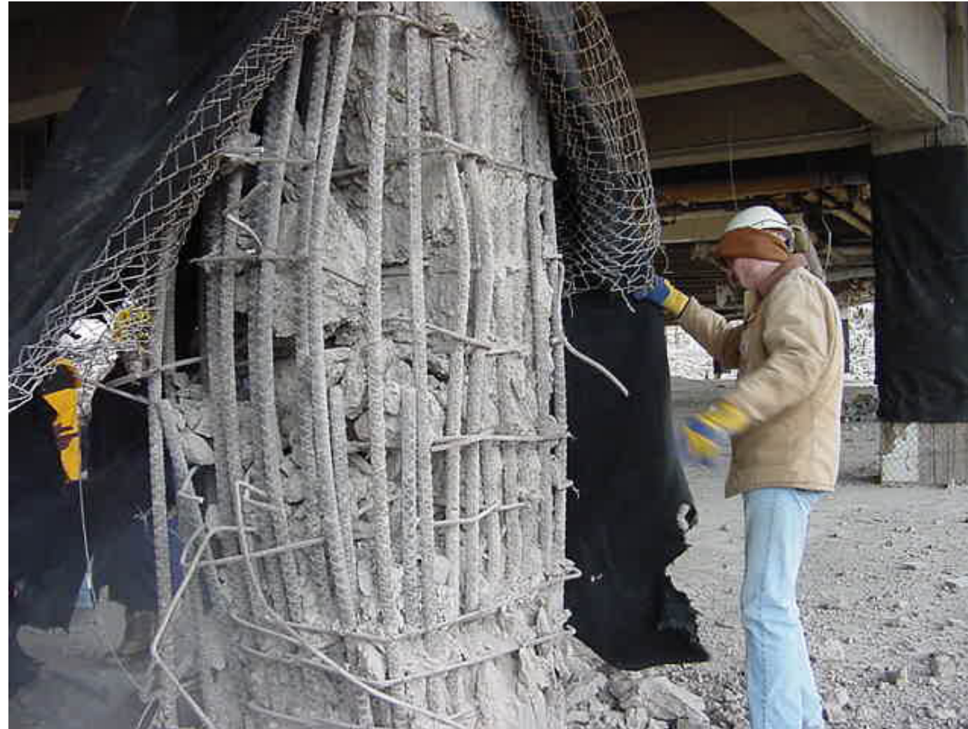
The column pictured shows the effects of the test blast. The blast caused the rebar within the column to vibrate and bend outwards allowing the concrete to pulverize.
