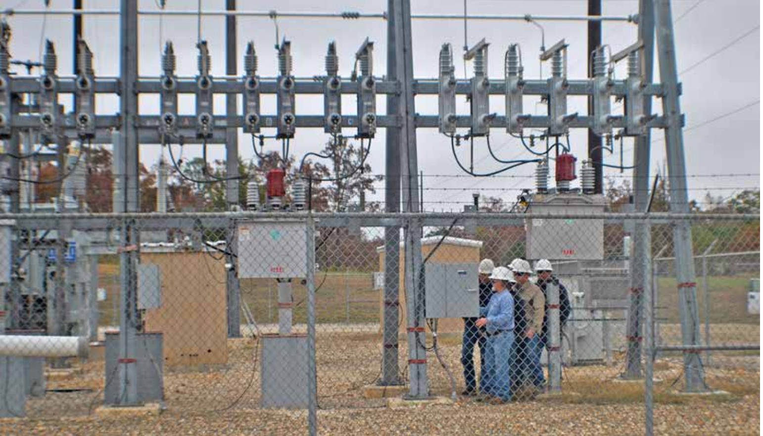
WFEC representative Tim Lisenberry explains some of the new features of the Hochatown substation to CEC employees. PHOTO/JENNIFER BOLING.
