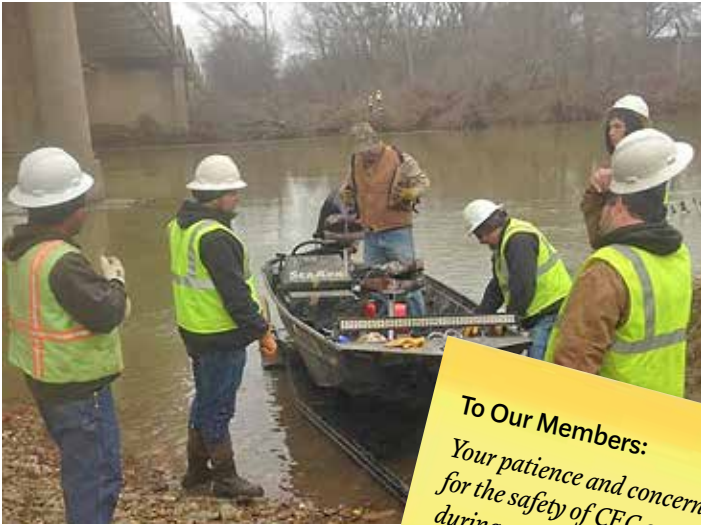
Choctaw Electric linemen prepare to ford the frigid waters of the Glover River following storms in December. Crew members raised 680 feet of submerged wire and reattached it to poles on either side of the stream. PHOTO/NORVIN GRAHAM
