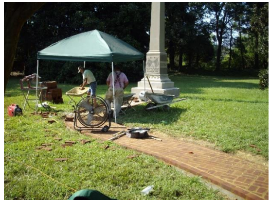
In August, Compatriot Tim Norman and his crew from Beneficial Masonry laid the sidewalk.
