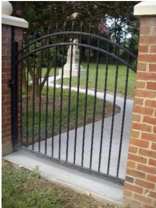
In July, Chuck Mihalcoe and ABBA Concrete poured the base for the walkway from the gate to the Soldier & Sailor's Monument.
