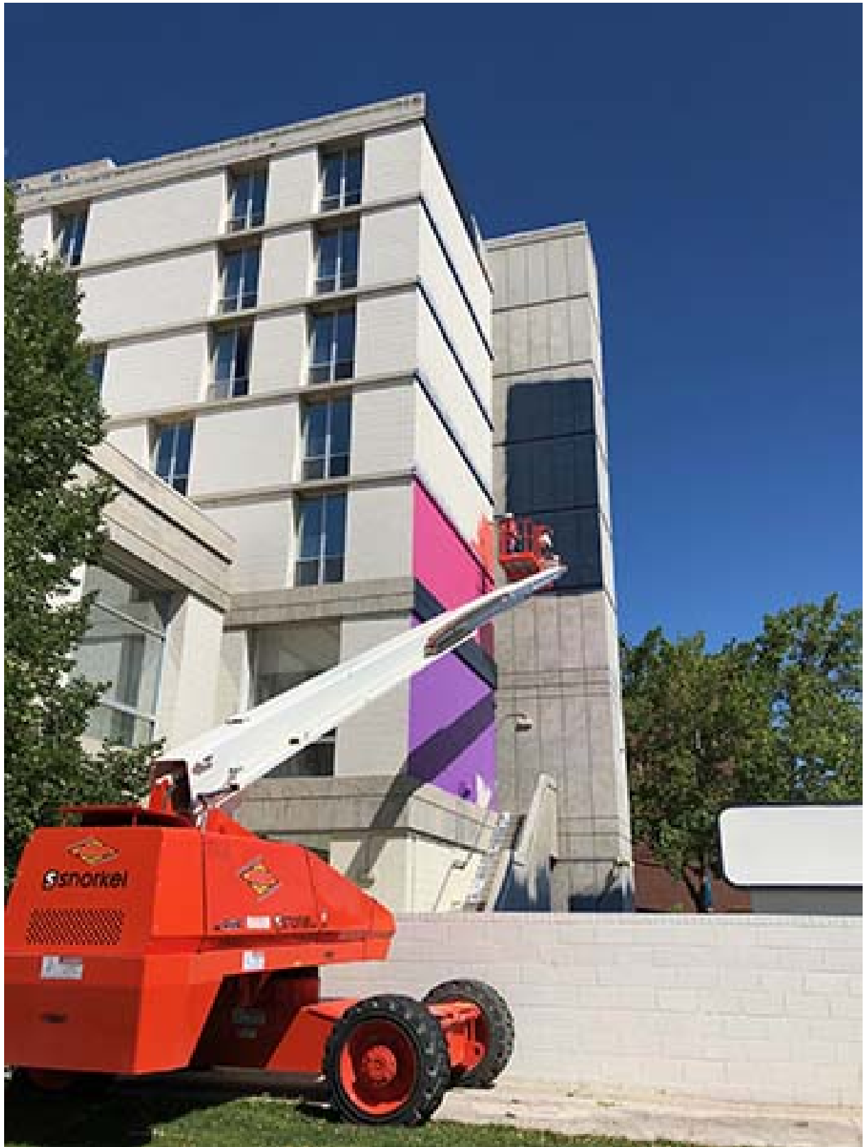
Artist Rafael Blanco begins work on a mural on the Sierra Hall building at the University of Nevada, Reno.
