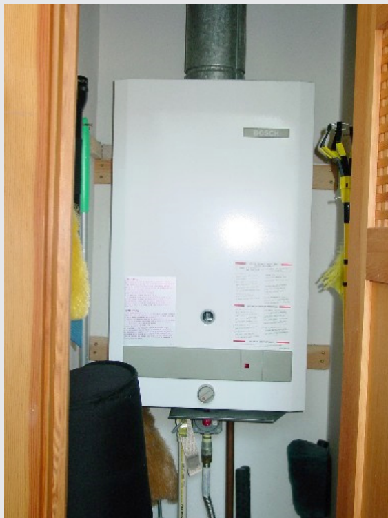
Gas-fired on-demand water heater. Photo: Oregon Department of Energy
