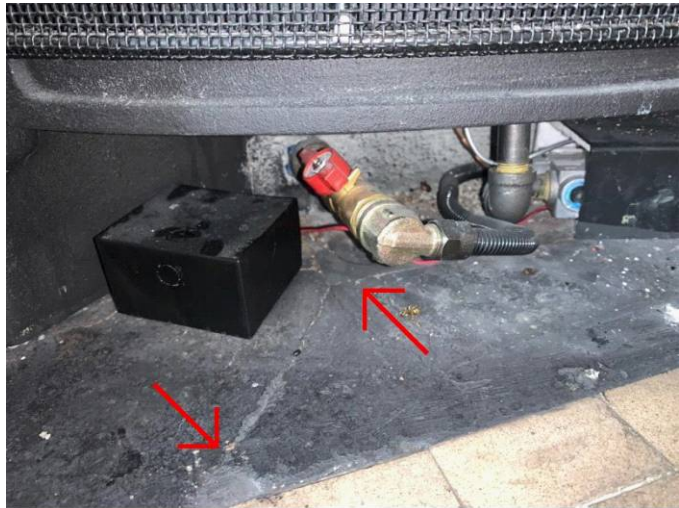
cracking of the hearth/firebox
