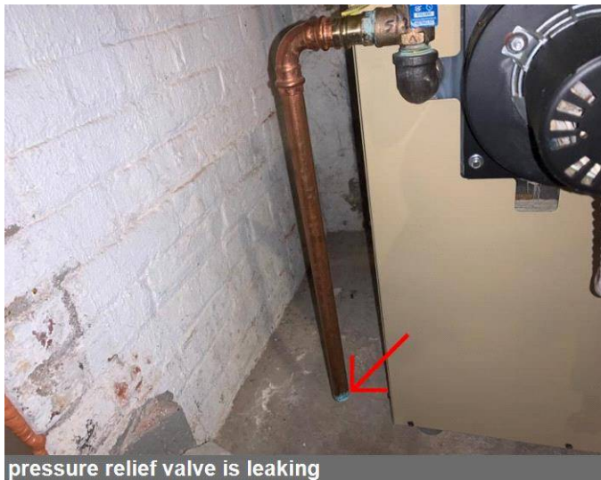
pressure relief valve is leaking
