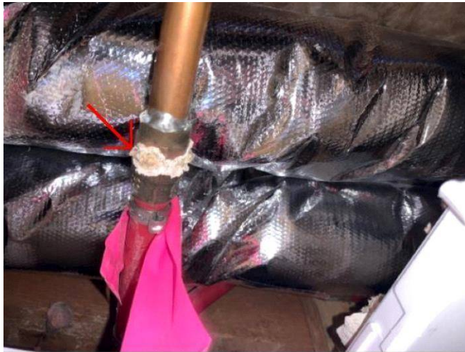
"pinhole" leakage from piping/fittings
