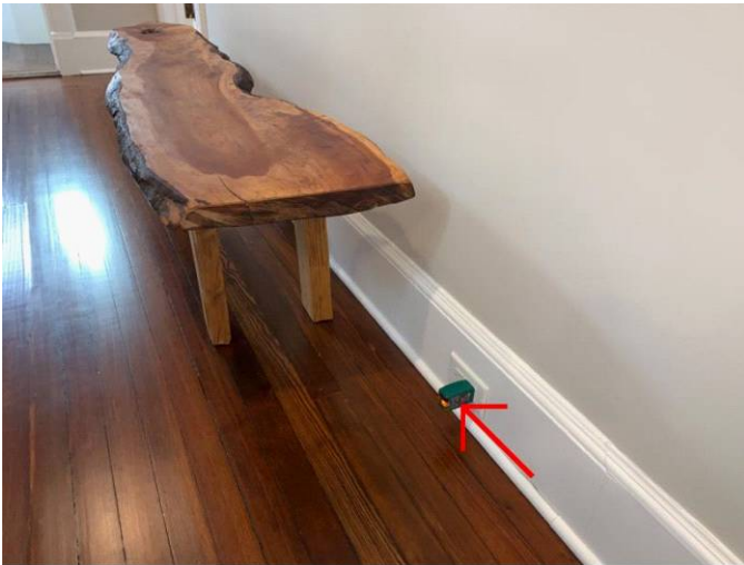
Ungrounded outlet/s detected
