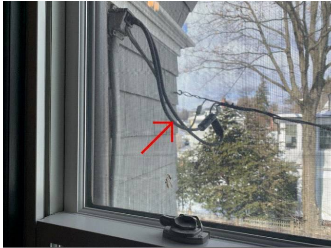
Too close to window | HAZARD
