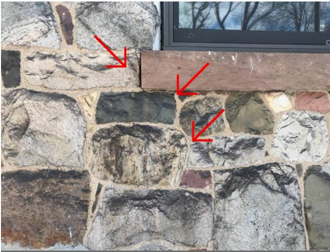
cracking of the mortar
