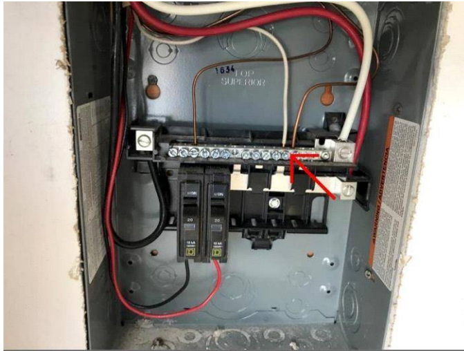
Improper wiring in panel | HAZARD
