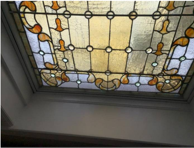
window units are damaged/broken
