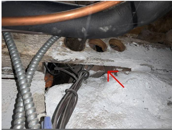
exhaust flue vent is not properly sealed
