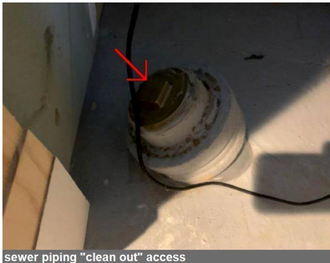
sewer piping "clean out" access
