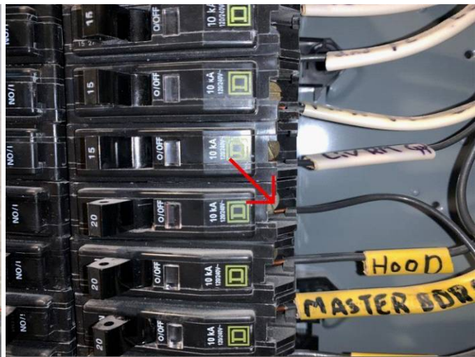
improperly sized over-current protection
