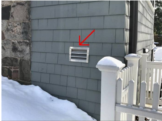
missing or defective flashings
