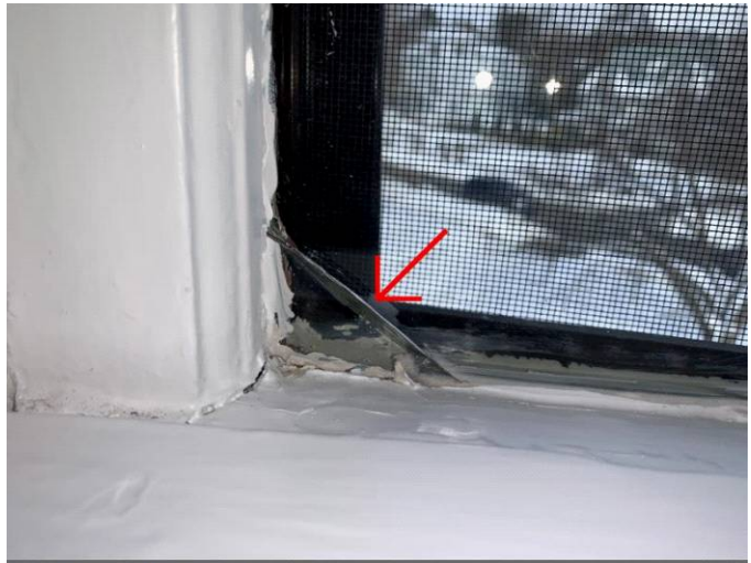
Cracked window glass
