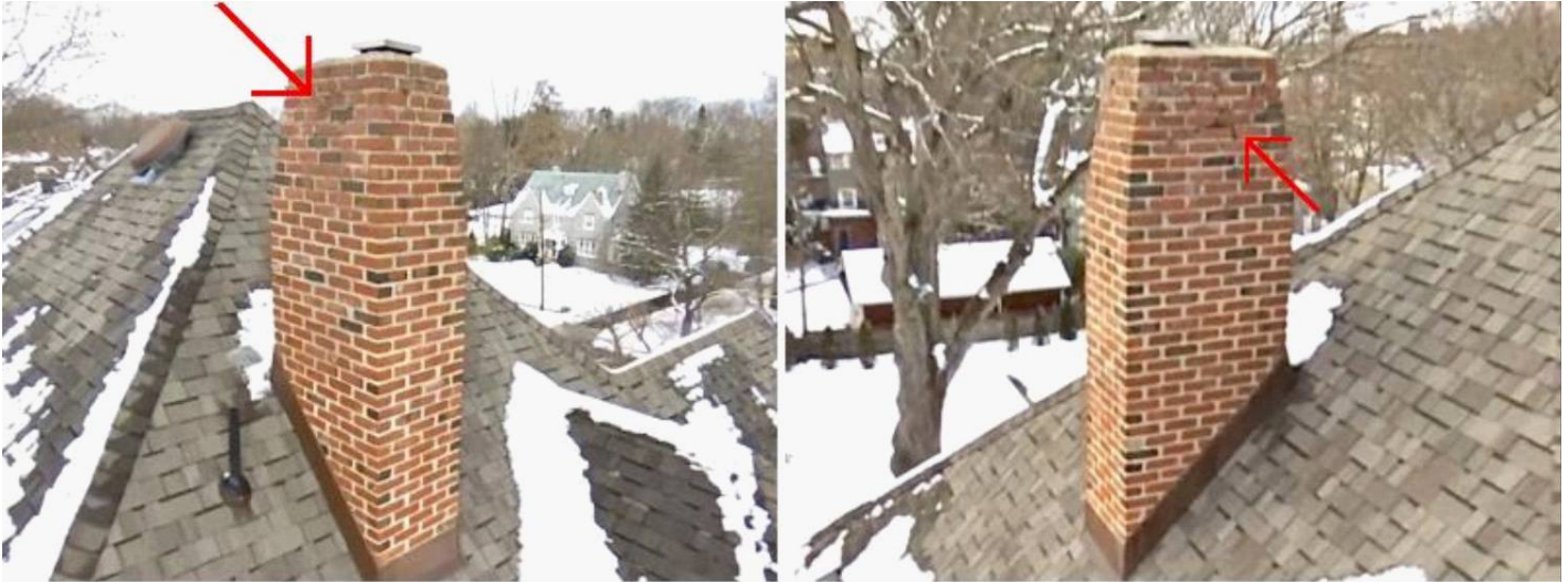
cracking of the masonry structure
