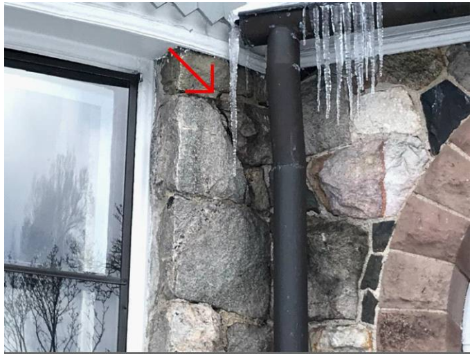
cracking of the mortar
