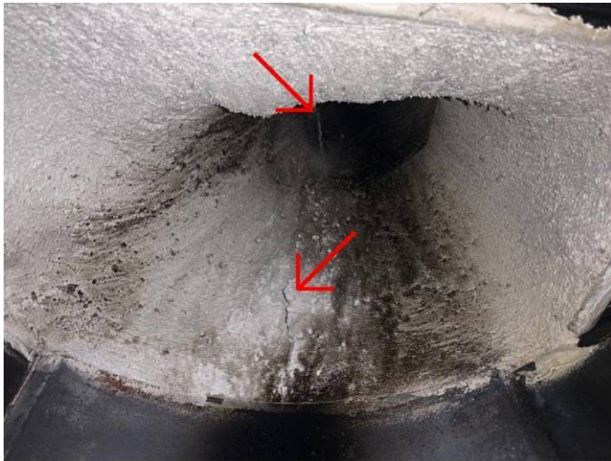
view of flue liner/smoke-chamber (cracked)
