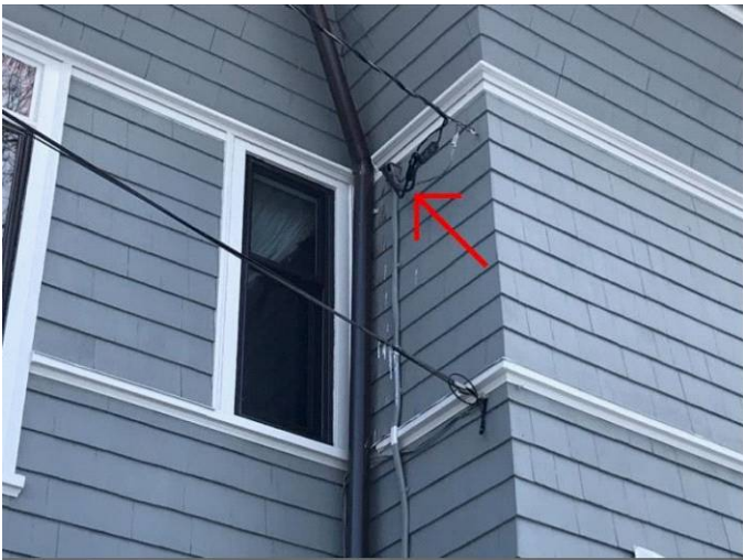
Too close to window | HAZARD
