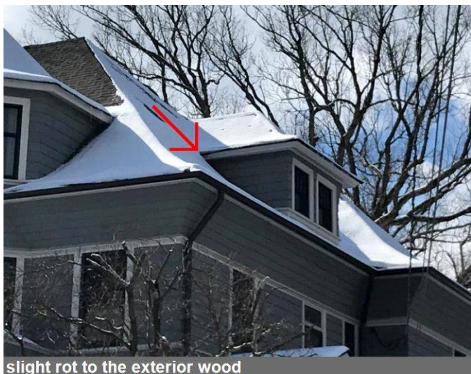
slight rot to the exterior wood
