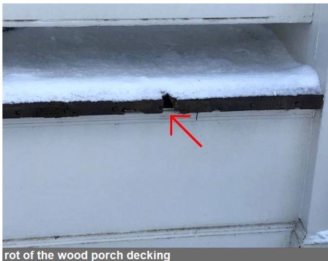
rot of the wood porch decking
