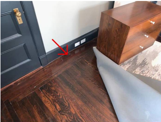
floor pops at the second floor
