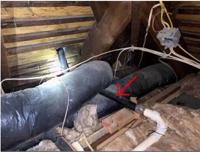
Back pitched vent pipe in attic area
