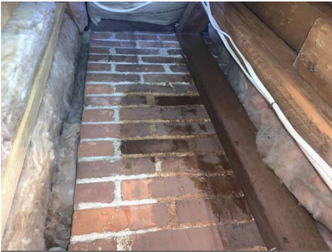
possible carbon staining
