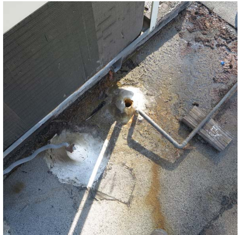
Disconnected condensate line
