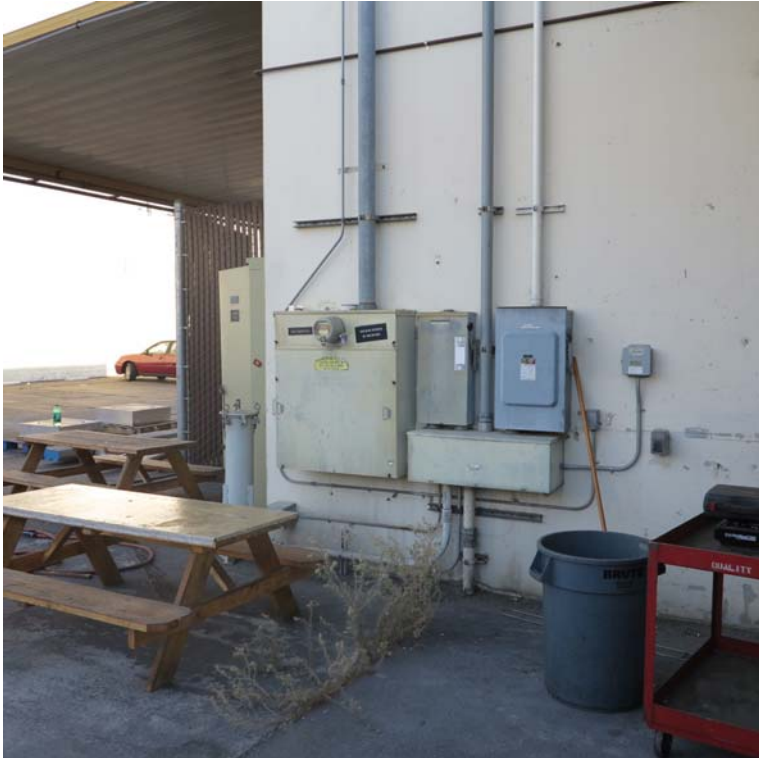
Service disconnect for 3310 - reads as 200 amp but is likely not correct
