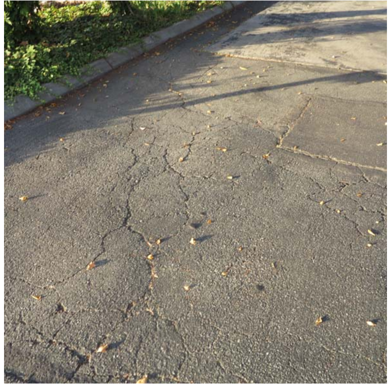
Front asphalt parking areas heavily "alligatored"
