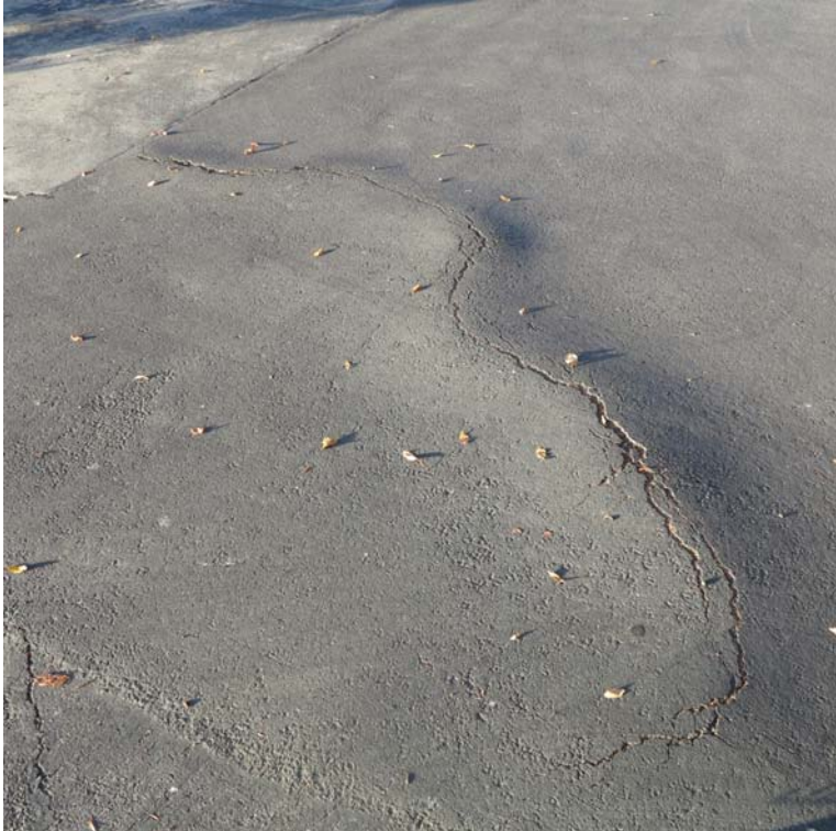
Tree root damage
