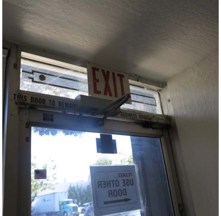
Locked door marked as an exit
