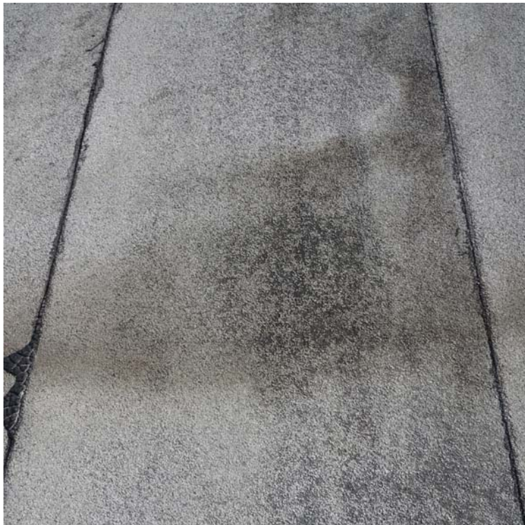
Roofing capsheet is wearing and losing protective granules
