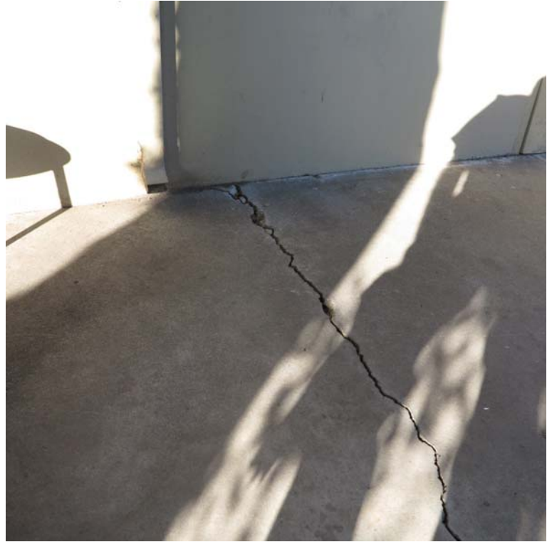
Tree root uplifting concrete walk way on east side of the bldg.
