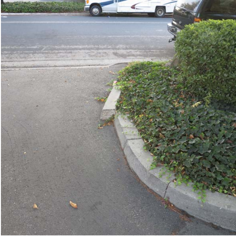
Landscape curb damaged
