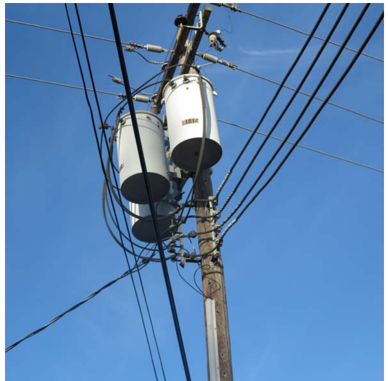
Pole mounted transformer in the NW corner of property
