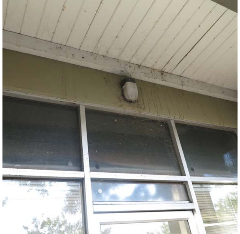
Typical lighting at entry canopies - likely do not illuminate parking adequately
