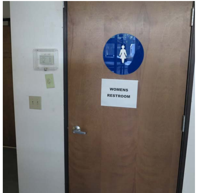
Missing braille signage at strike side of the door
