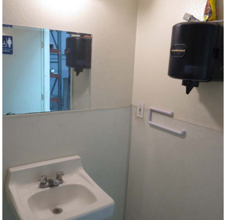
Mirror mounted too high
