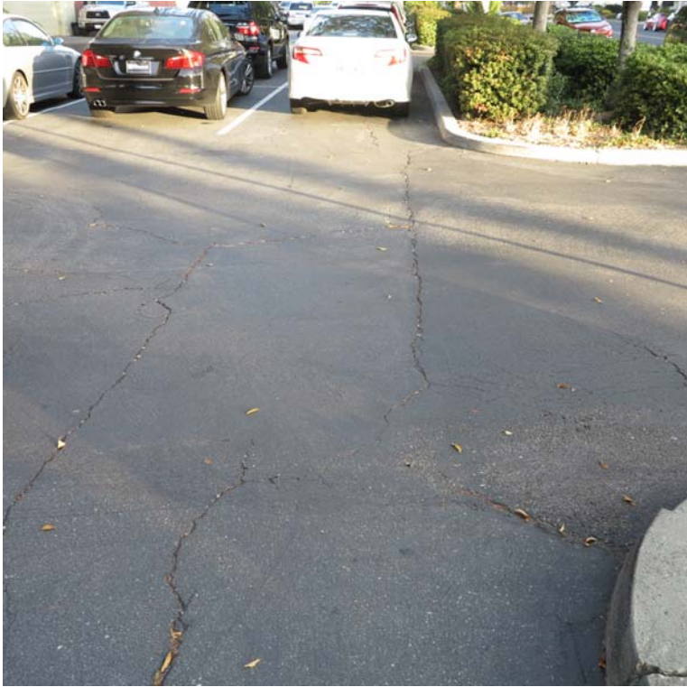
More asphalt damage in front parking
