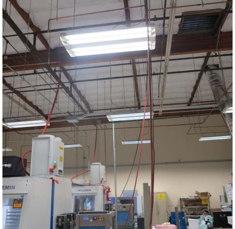
Suspended industrial fluorescent fixtures in 3310
