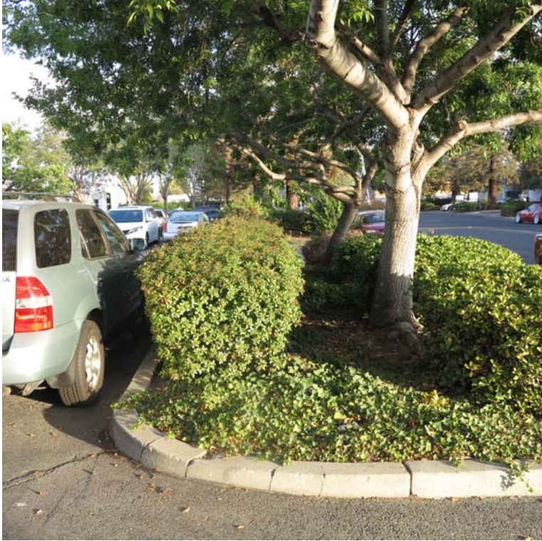
Tree root damage at curb and asphalt
