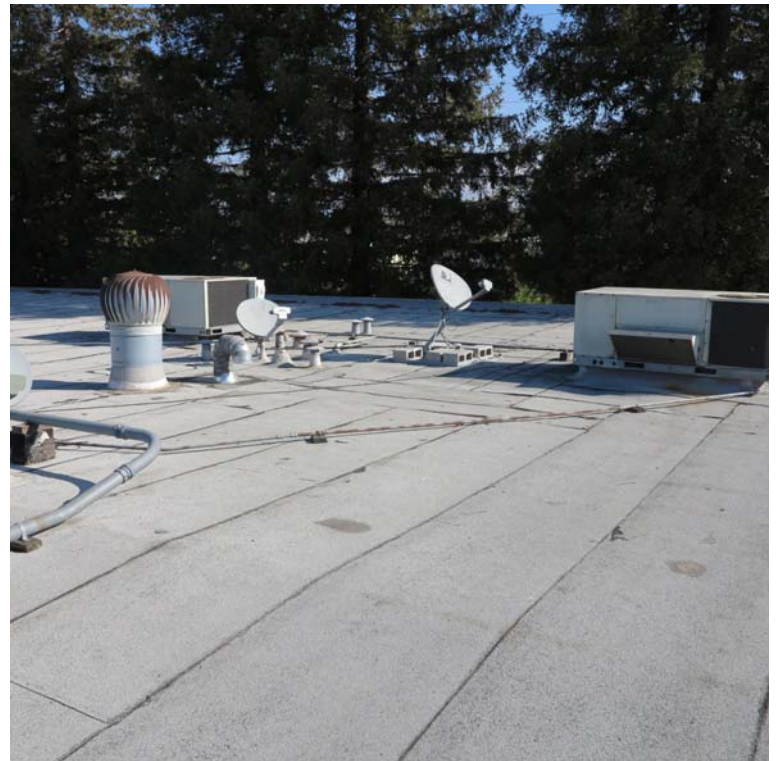
AC units over 3310
