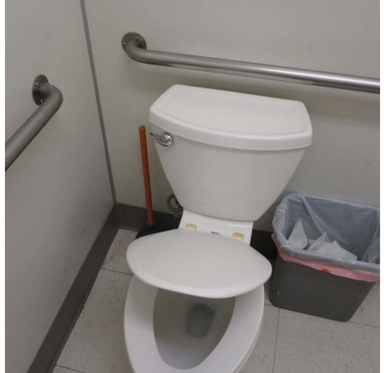
Flush control on the wrong side of the toilette fixture
