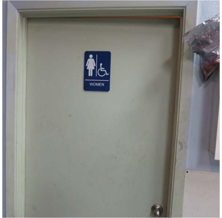
Incorrect signage and door hardware
