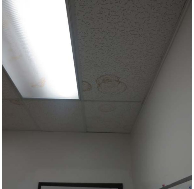
Stained ceiling tile -roof leak likely cause
