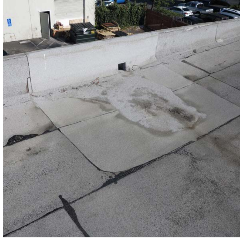
Evidence of ponding
