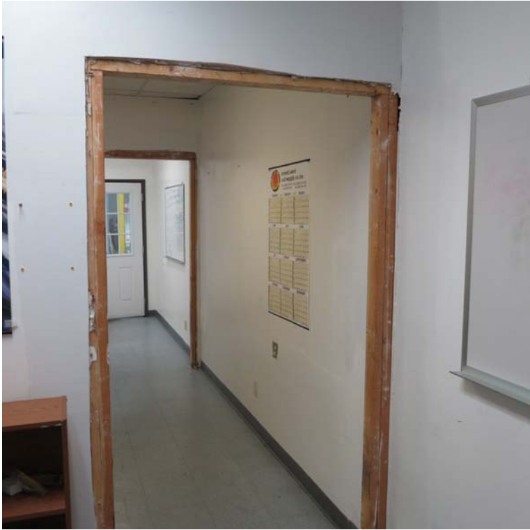
This work was allegedly done with permit, cosmetic work unfinished
