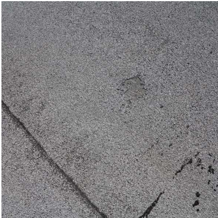
Fibers showing in the cap sheet here and there
