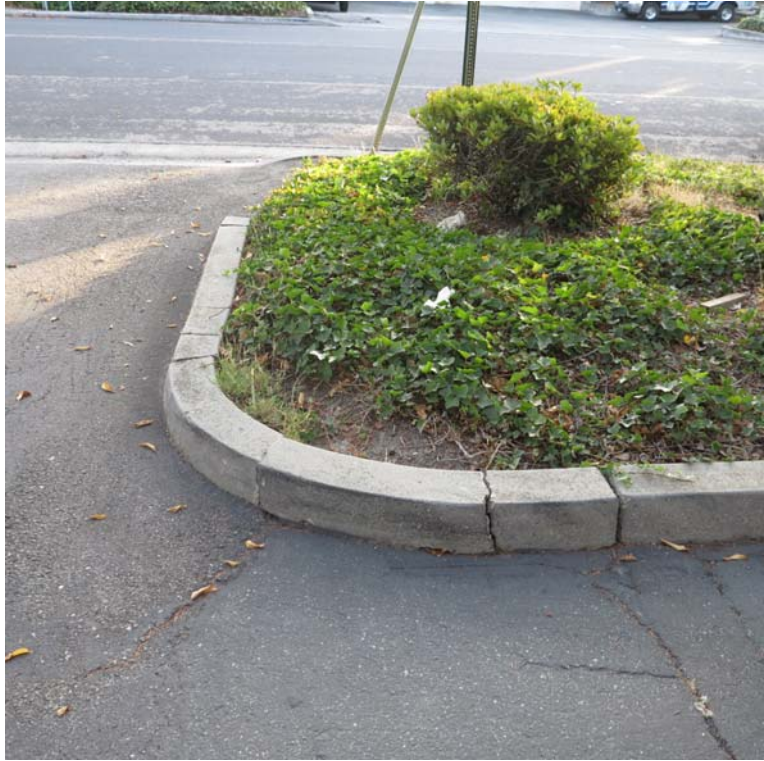
Landscape curb damaged
