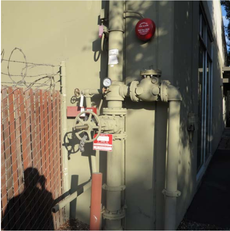
Sprinkler riser at the SE corner of the bldg.
