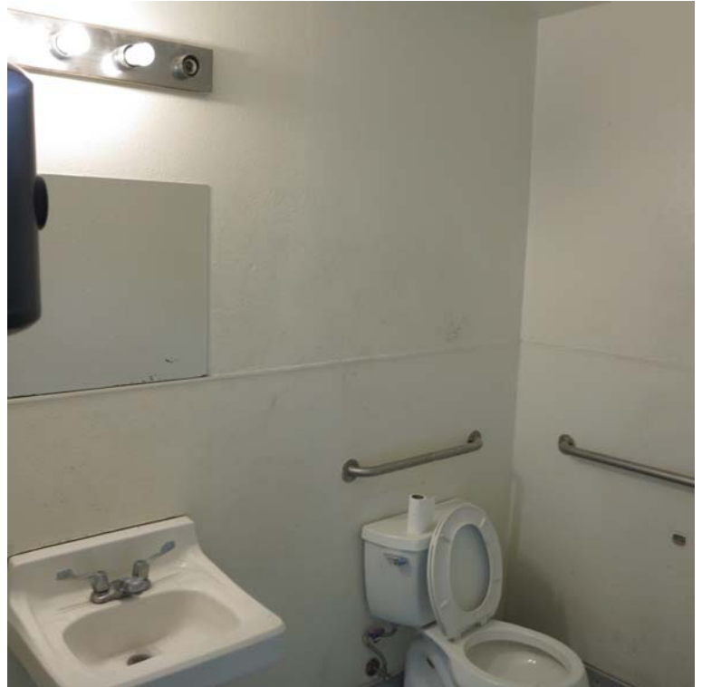
Mirror mounted too high
