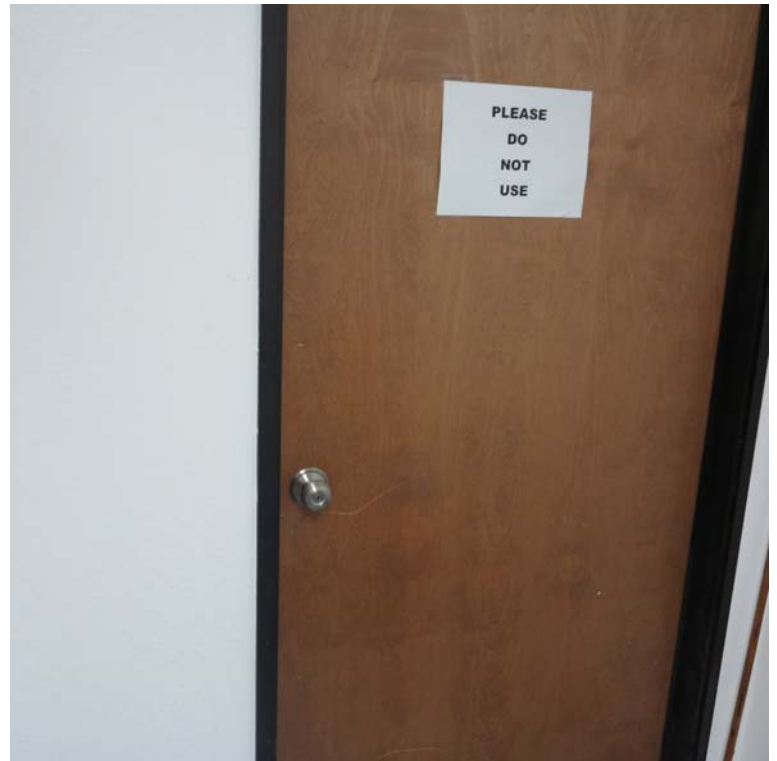
Unused restroom has improper (round) hardware
