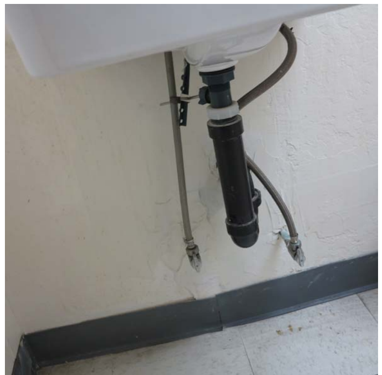
Uninsulated hot water and waste line
