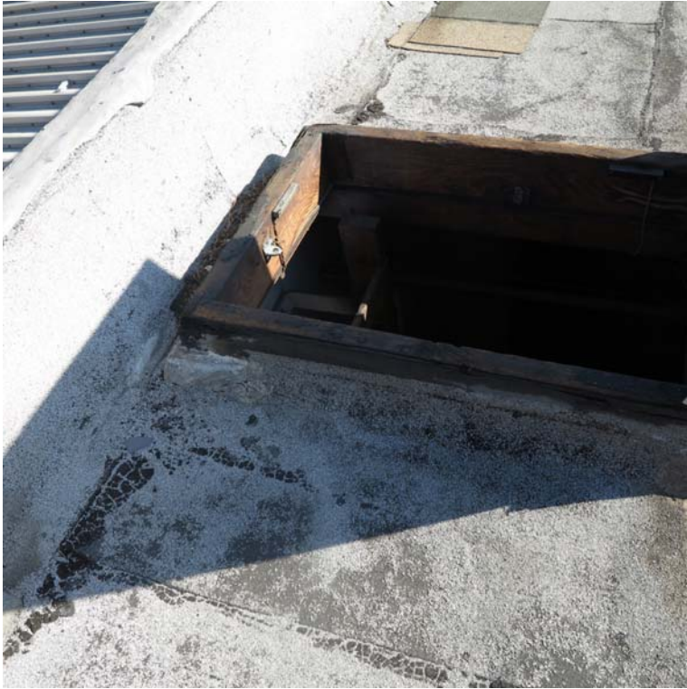
Substandard and dangerous roof hatch
