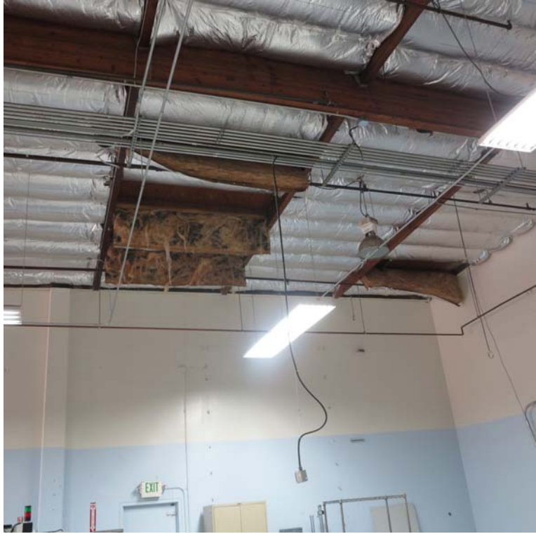
More falling insulation
