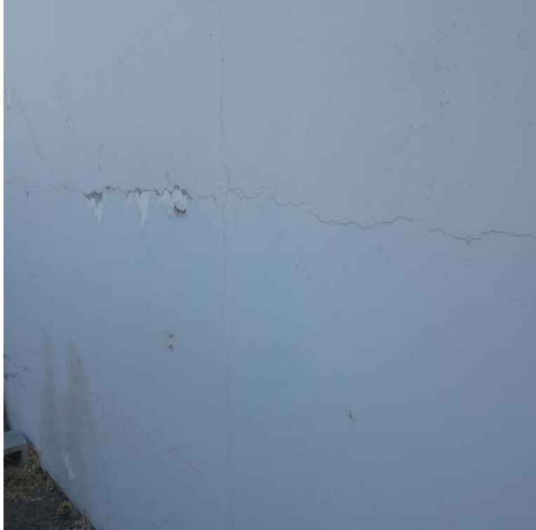
Tiny fractures in the west wall of 3310, not serious.
