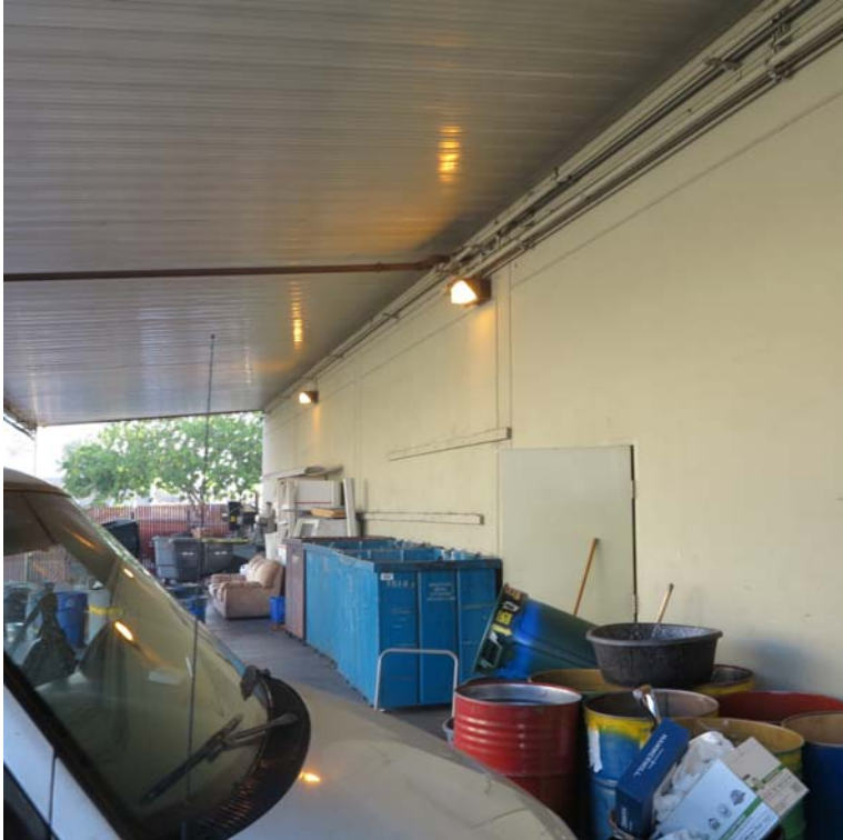
Wall pack lighting at 3314
