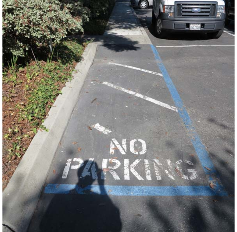
Ramp# 2 is not compliant
