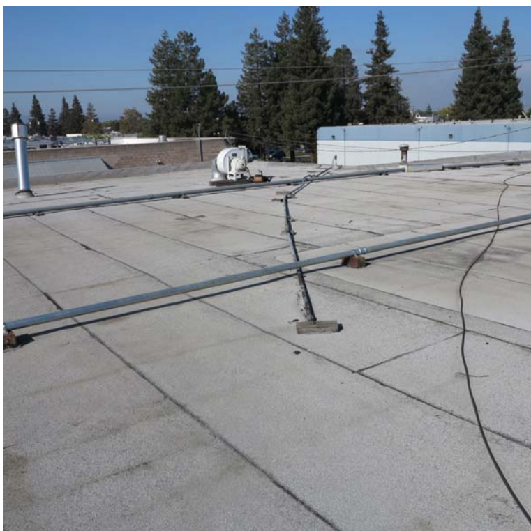
Abandoned lines, multiple occurrences
