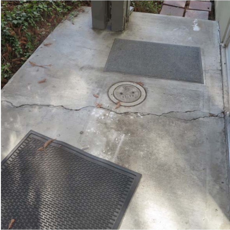
Fracture at 3310 entry where south part of the walkway appears to be subsiding
