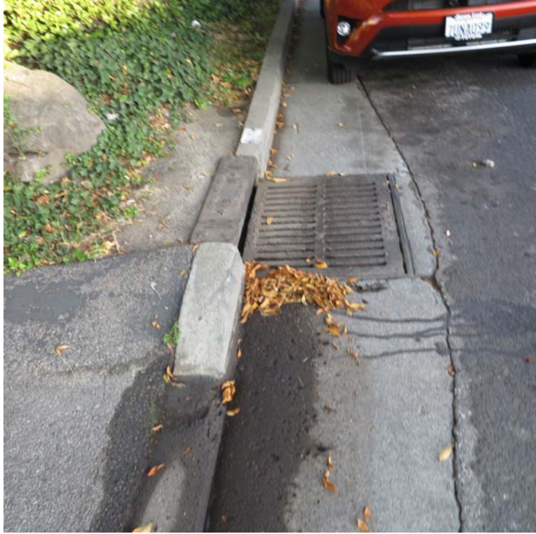
Street catch basin
