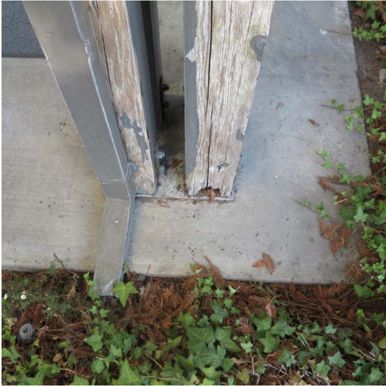
Southmost vertical wood members are dry rotted.
