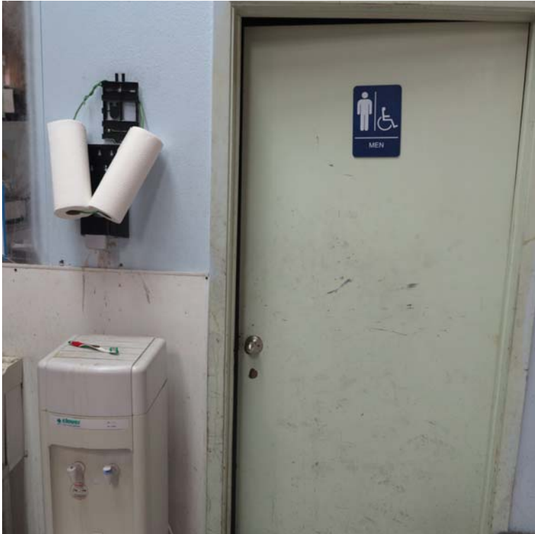
Incorrect signage and improper door hardware
