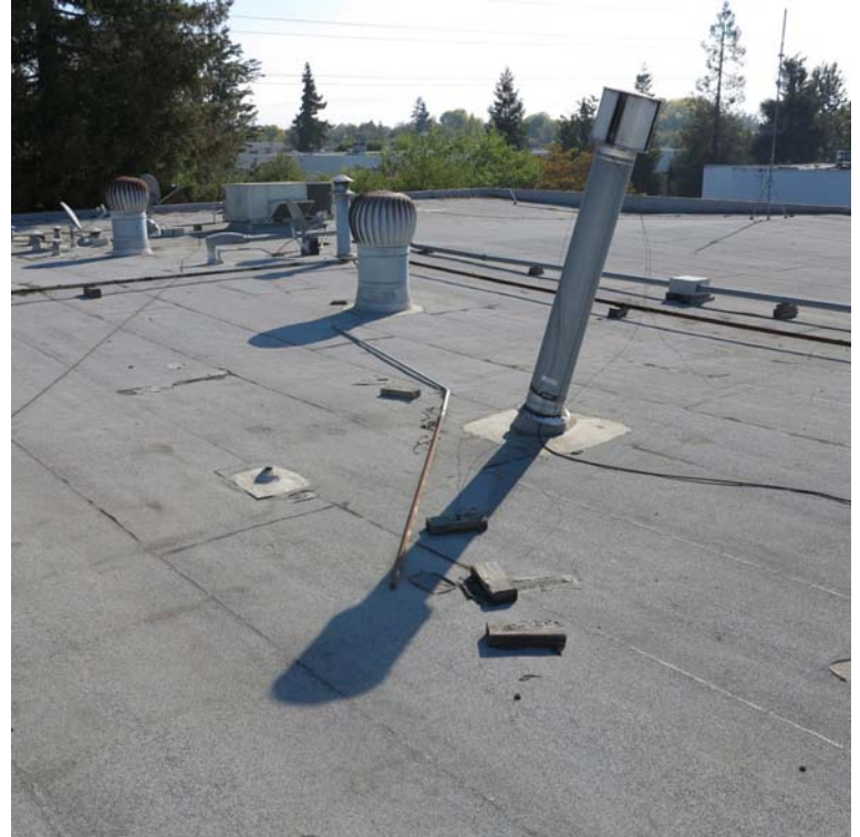
Leaning vent above 3310
