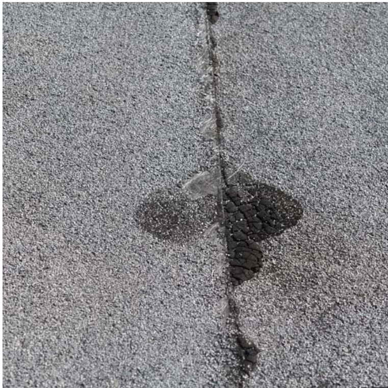
Fibers exposed here and there
