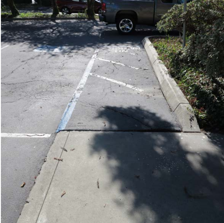
Ramp # 1 is not compliant
