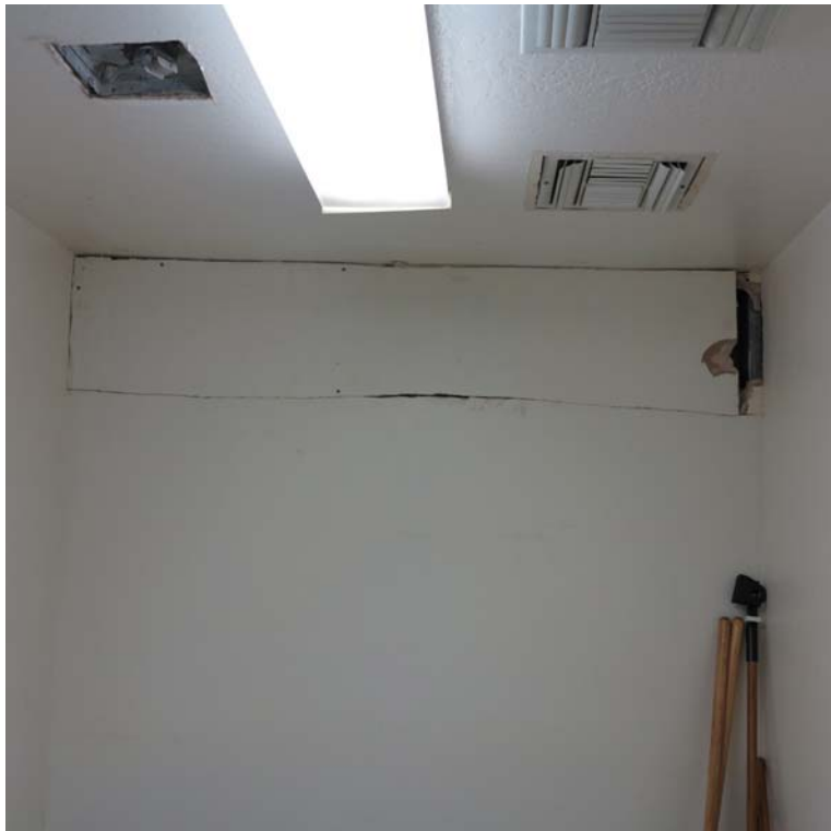
Drywall damage in one of the restrooms
