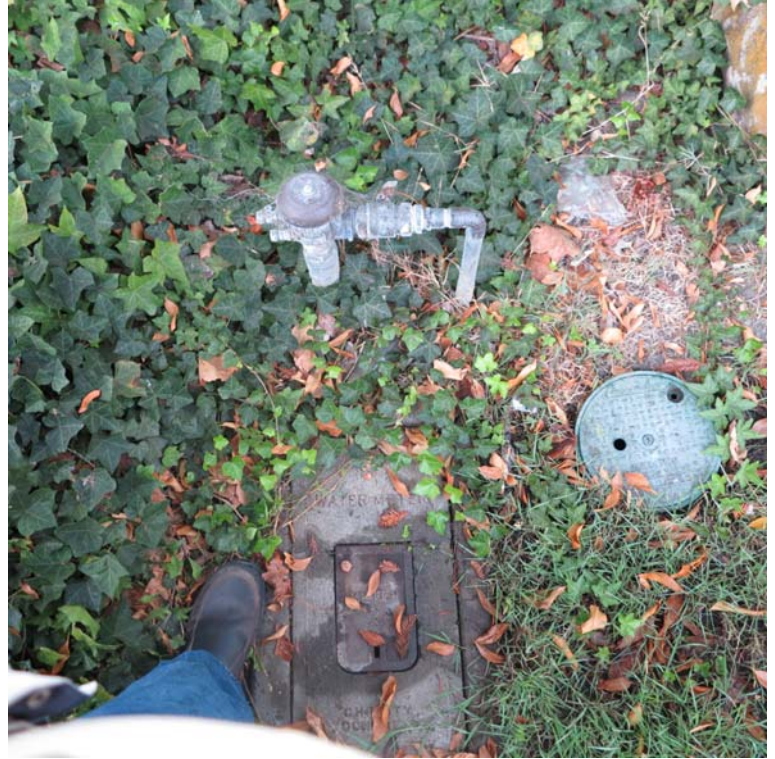
Water meter, supply and backflow preventer
