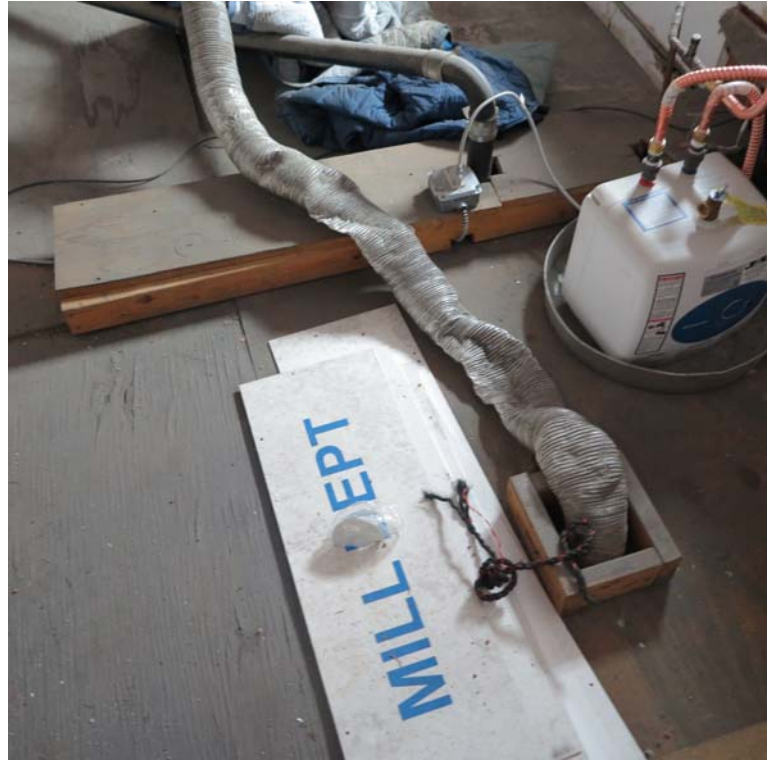
Crushed RR vent at 3320 shop restrooms
