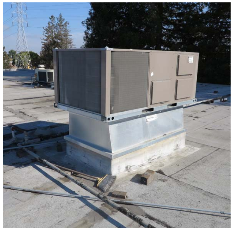
Relatively new AC unit, downflow, unusually tall curb
