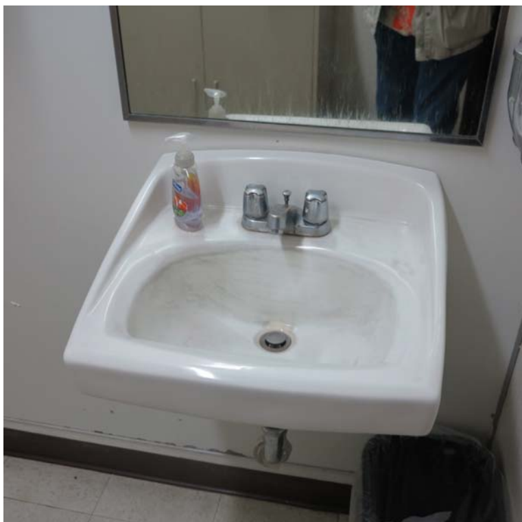
Incorrect faucet style (requires grasping)
