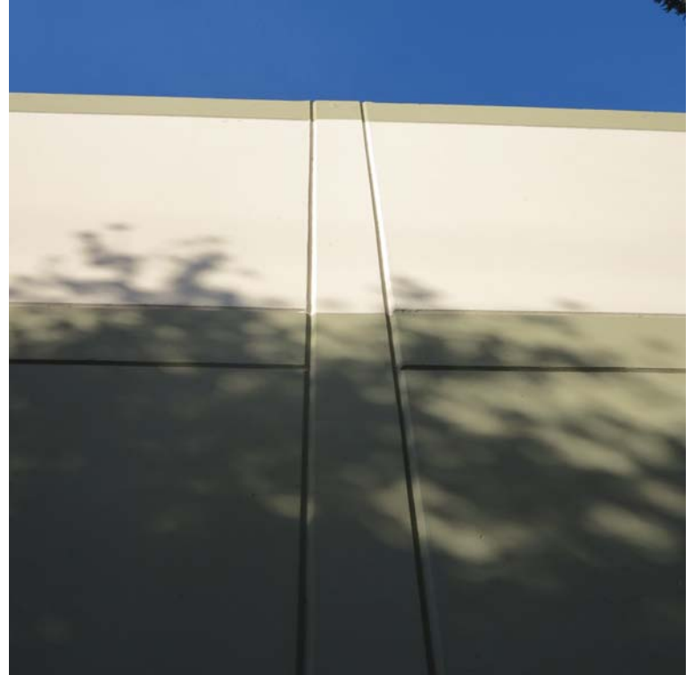
Typical panel joints at exterior - all are even and packed with caulk
