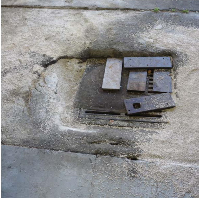
Failure at storm drain- appears to have been this way for some time
