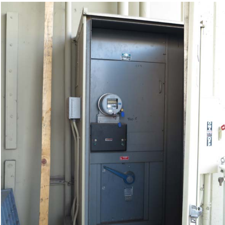
Main disconnect for 3314 is 600 amps @240v
