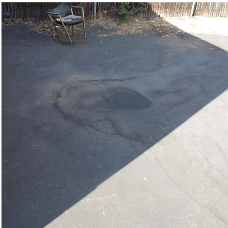
Some ponding of rainwater
