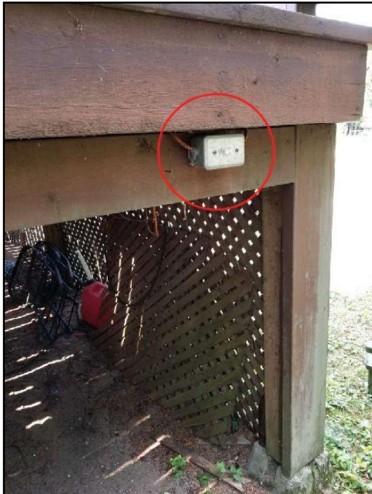
79. Extension cords for exterior outlets...
