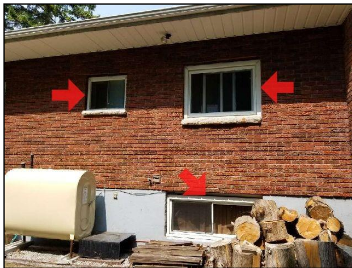
27. Paint and Caulking - deteriorated / missing
