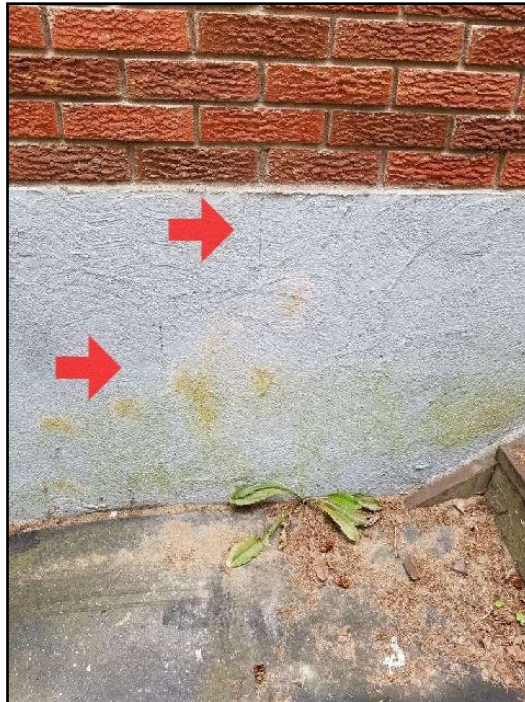
60. Typical minor cracks
