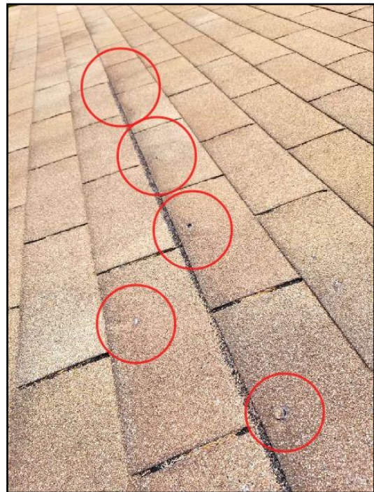
9. Missing, loose or torn
