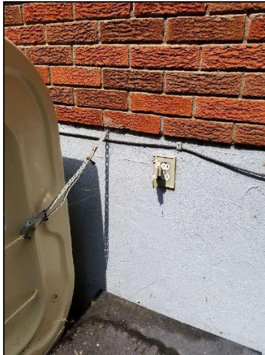
85. No GFCI/GFI (Ground Fault Circuit...
