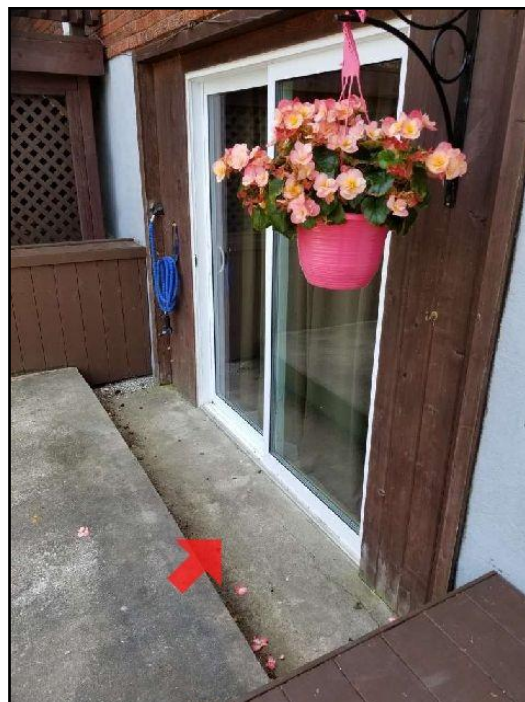
38. Door threshold missing, too low, not...
