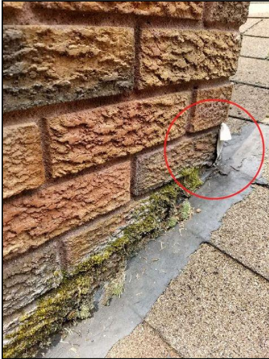
17. Damage, loose, open seams, patched
