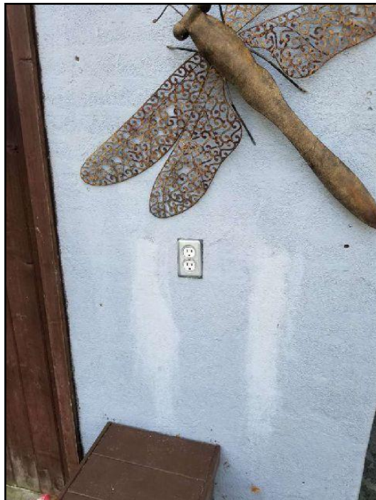
83. No GFCI/GFI (Ground Fault Circuitit...
