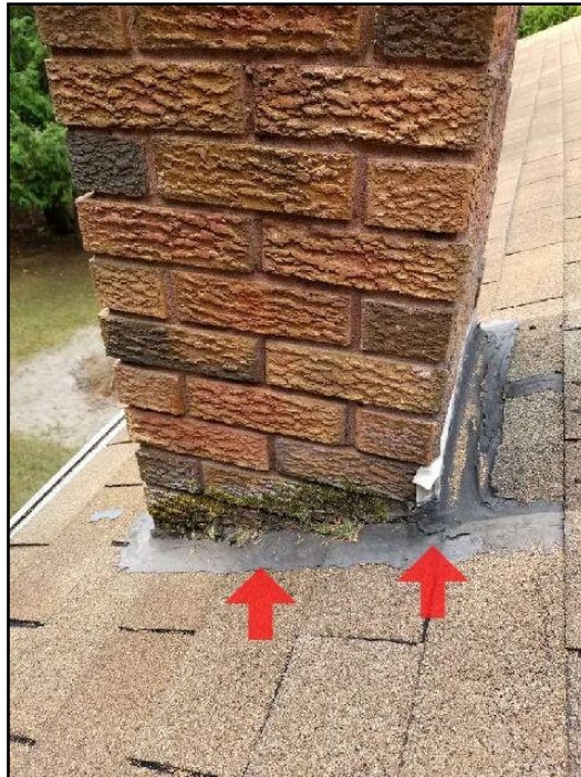
19. Damage, loose, open seams, patched
