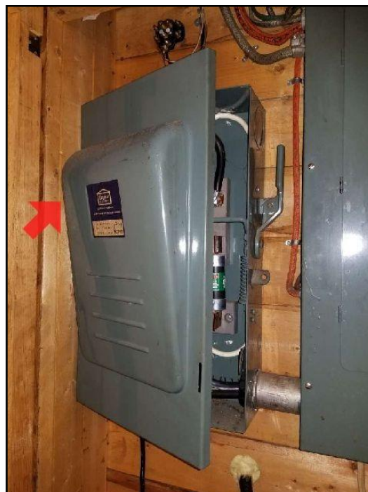
75. Box location poor
