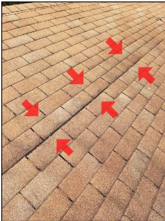
8. Missing, loose or torn
