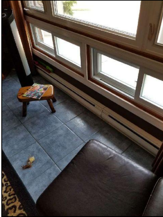
89. Electric baseboard heaters
