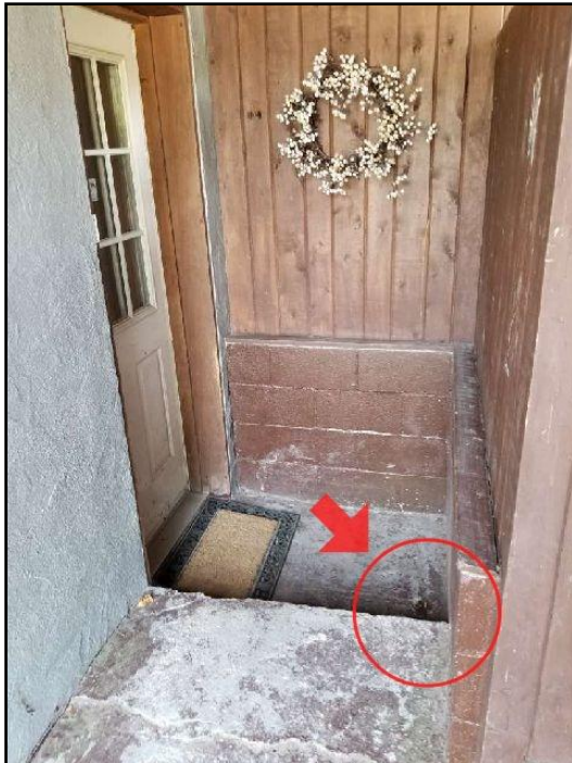
36. Drains missing, clogged or undersized
