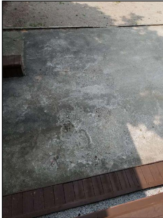
39. Cracked or damaged surfaces
