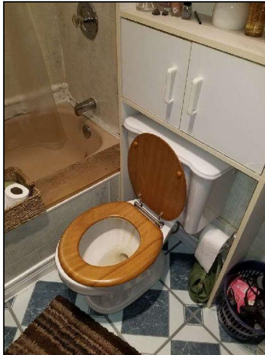
119. Obstructed or weak flush
