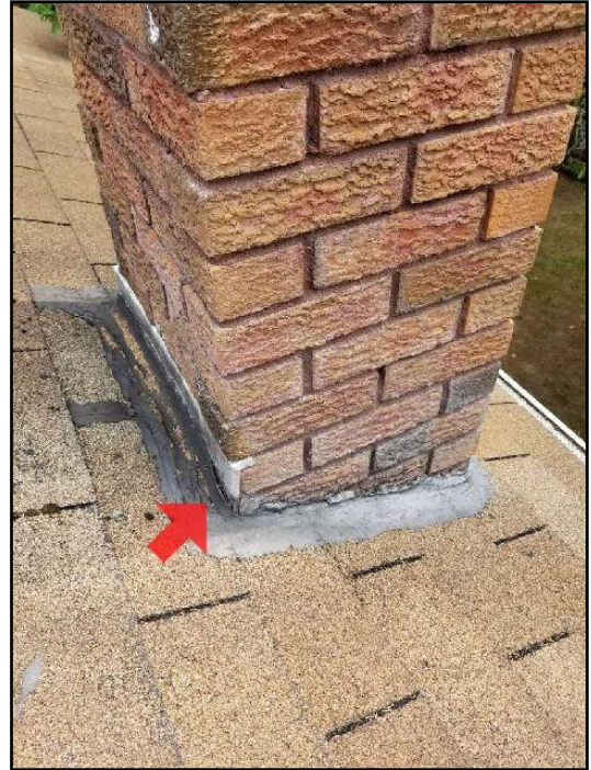
18. Damage, loose, open seams, patched
