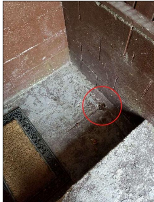
37. Drains missing, clogged or undersized
