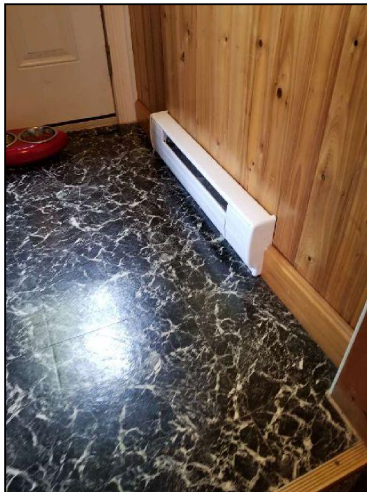
91. Electric baseboard heaters
