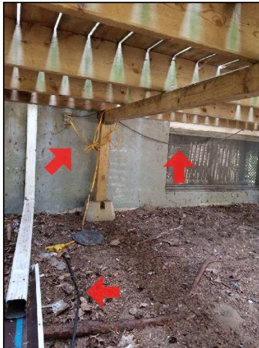
81. Extension cords for exterior outlets...
