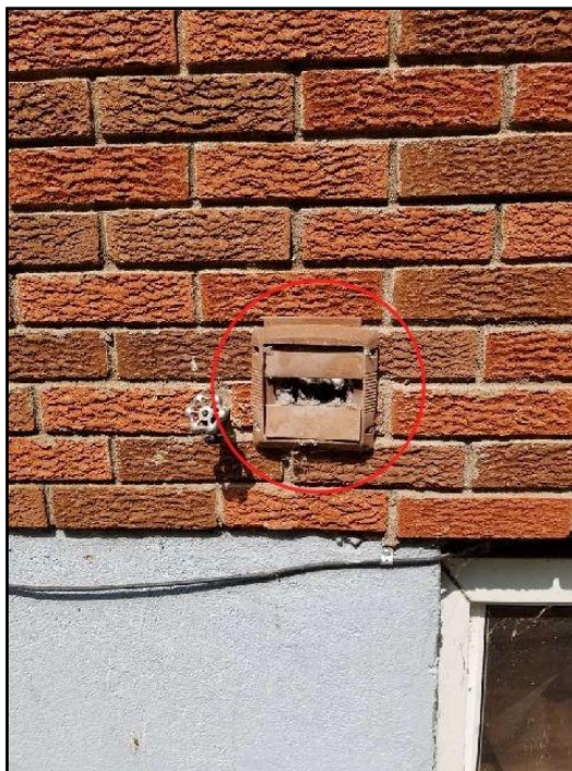
26. Flashings incomplete or ineffective
