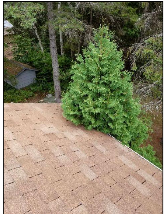
12. Tree branches touching roof
