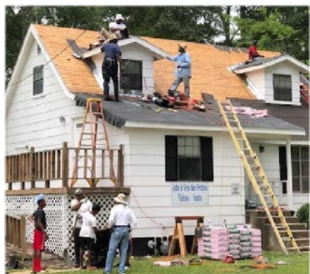
Volunteers from First Baptist Church of College Hill, Tampa, FL replaced roofing on John & Vera Mae Perkins Visitors Center.
