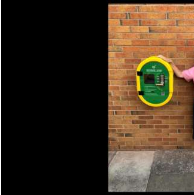
Defibrillator Installed at Methodist Church in Aintree Village
