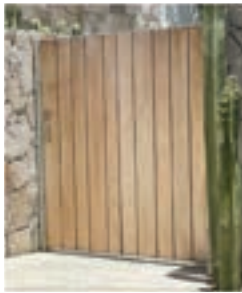
EXTERIOR ENTRY DOOR
