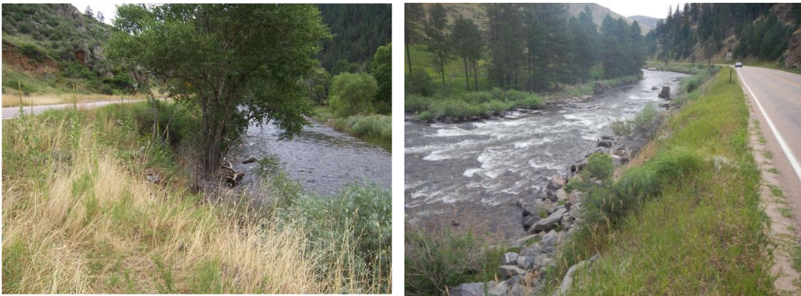
Figure 3.8: Highway 14 road fill encroachment in the riparian floodplain is common in the Canyon zone.
