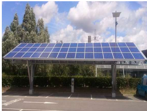
Canopies with solar panels, that will help have own sources of power
