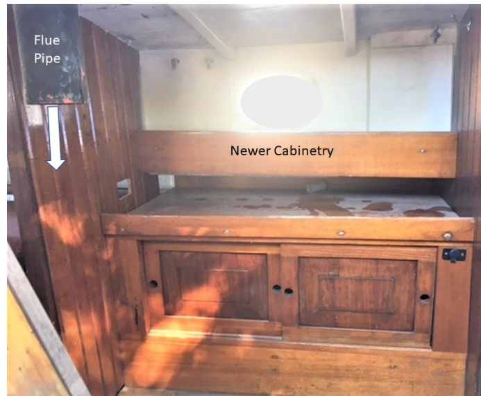
Figure 4: With the flue pipe misaligned, there was no place to mount her Shipmate #1 stove
