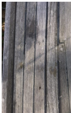
Figure 6: Damaged teak deck sections required challenging repair methods
