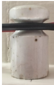
Figure 11: The foremost cabin roof support contained a number of knob and tube ceramics
