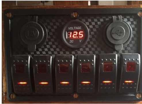
Figure 14: The new breaker panel offered many features not even invented for the old panel
