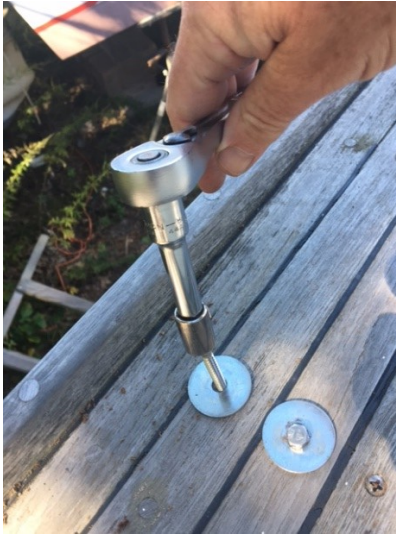
Figure 7: Deck repairs utilized long screws and fender washers to unwarped deck sections
