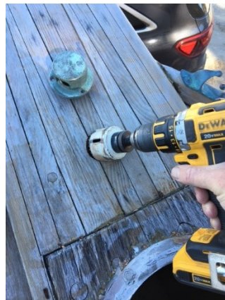
Figure 17: Installation of the antique hawser pipe was straightforward with a drill hole saw
