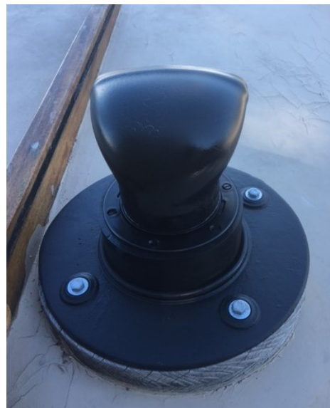
Figure 21: The addition of a rubber cowl turned the water deck iron into a ventilator
