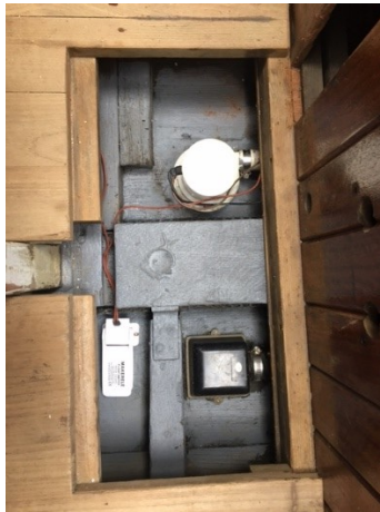
Figure 15: The automatic bilge pump and the intake for the manual Guzzler share bilge space
