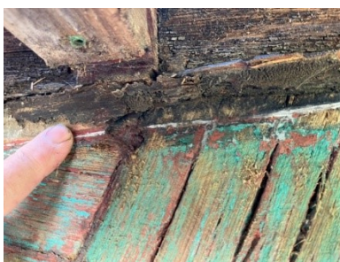
Photo 2: No stopwaters where they should have been.
