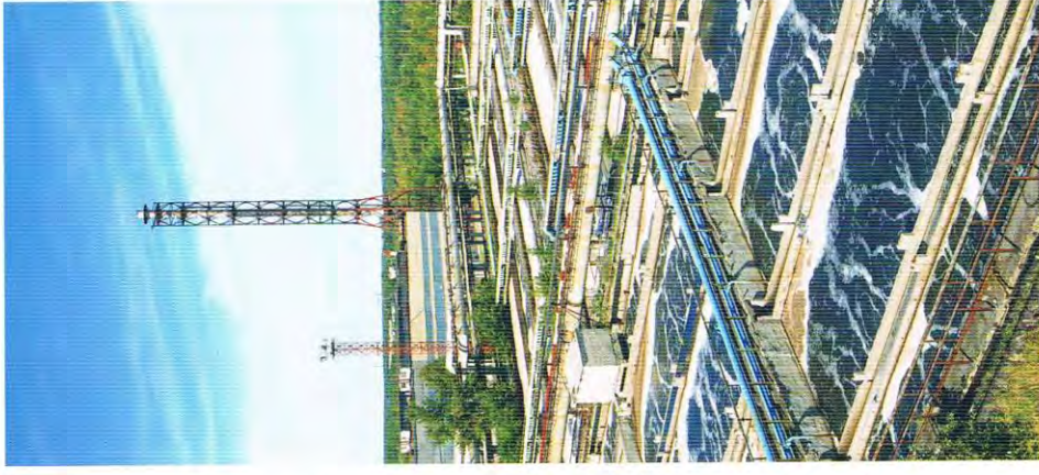
Water treatment facility
