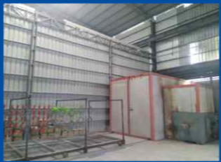
大型烤漆房 Large paint baking room
