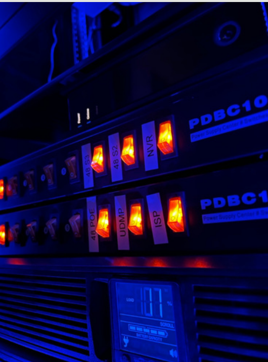
Power Distribution + Surge Protection
