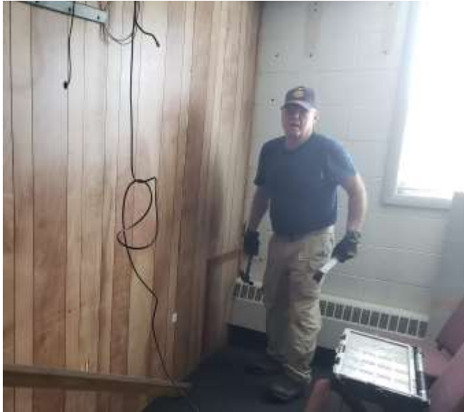
Comrade Kimball Thompson prepares to begin the demolition of the existing wall.
