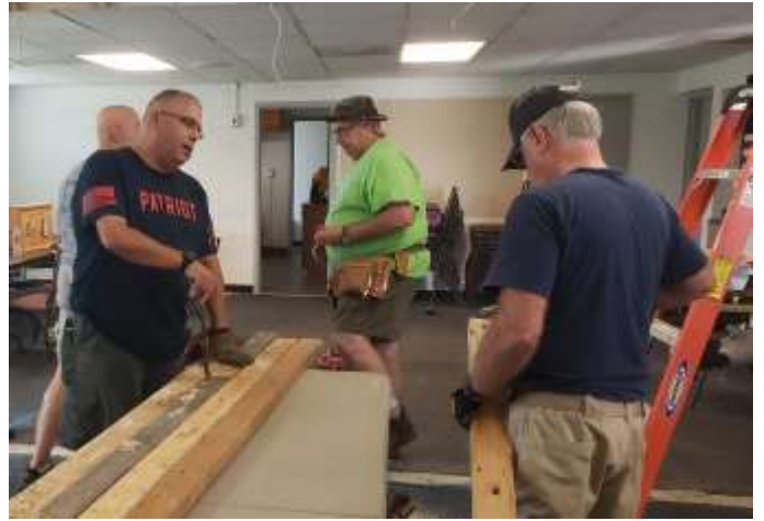
Comrade Tony Affa prepares removed wooden studs for reuse in the creation of the partition support frame.
