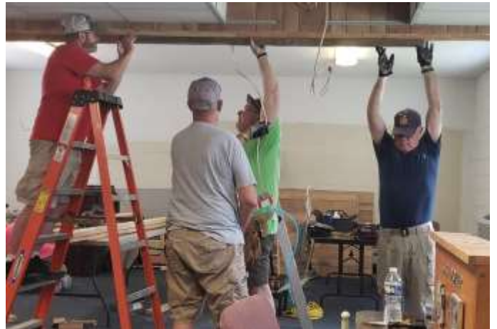
Post volunteers create the partition support frame from recycled studs from the removed wall.
