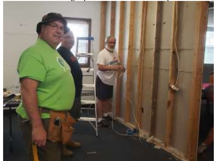
VFW Post 2894 member Frank Sgromolo, Tony Affa and Jim Keiper initiate demolition of the existing wall.
