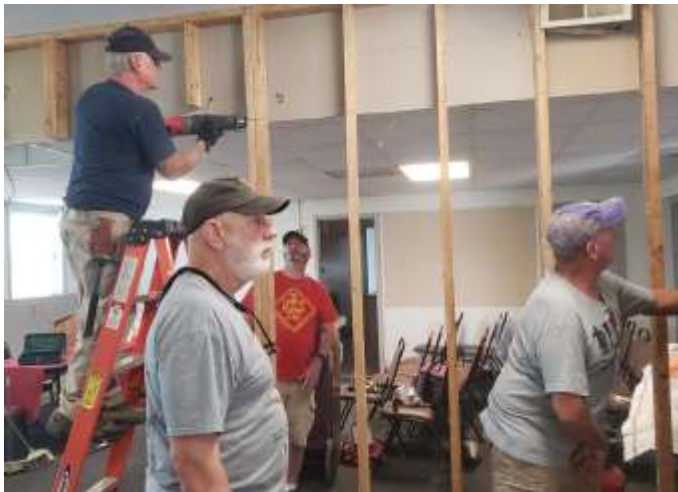
Comrade Kimball Thompson uses a saws-all saw to remove existing support wall studs as other volunteers assist.
