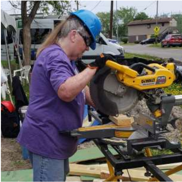
VFW Post 2894 Auxiliary member Sandy Dunbar trims lumber for a housing project.
