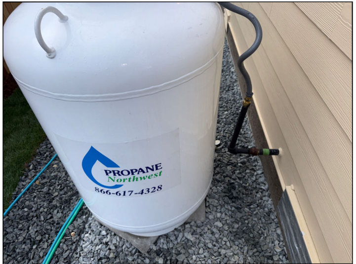
The propane tank was located on the east side of the home.
