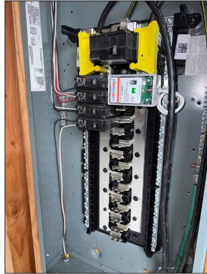
All of the circuit breakers appeared serviceable.
