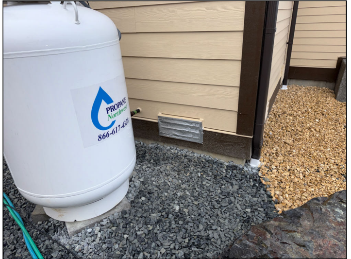
The crawlspace vent at the NE corner of the home has been covered over with foil faced ducting tape. This is not typical and should be removed or repaired as needed.
