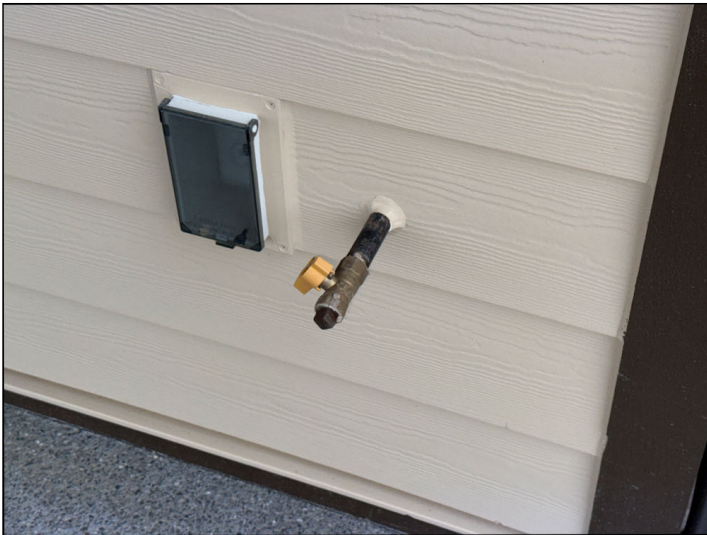
Gas lines have been installed to the back patio for future gas appliances.
