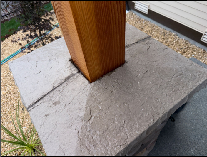
Caulking missing around the front porch post. Currently, water will travel down the post and get trapped inside the brick column.
