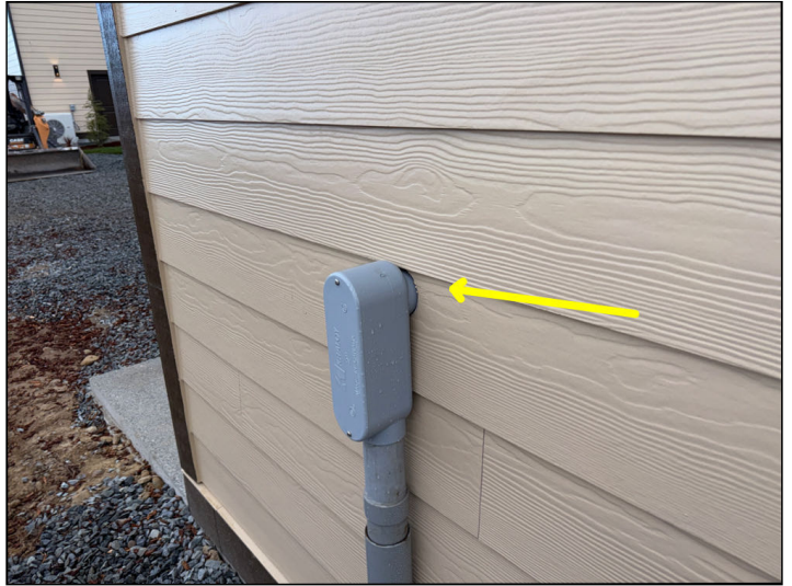
Recommend caulking around doors, windows and pipe penetrations as necessary where cracks or gaps exist.
