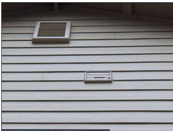
Peeling paint noted on the upper exhaust fan vent hood on the east side of the home.
