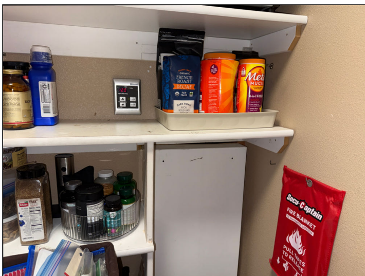
South water heater set at 120 degrees.
