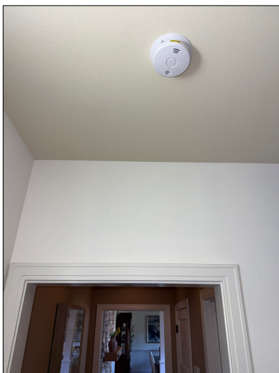
First floor CO and smoke detector noted in mudroom hallway.
