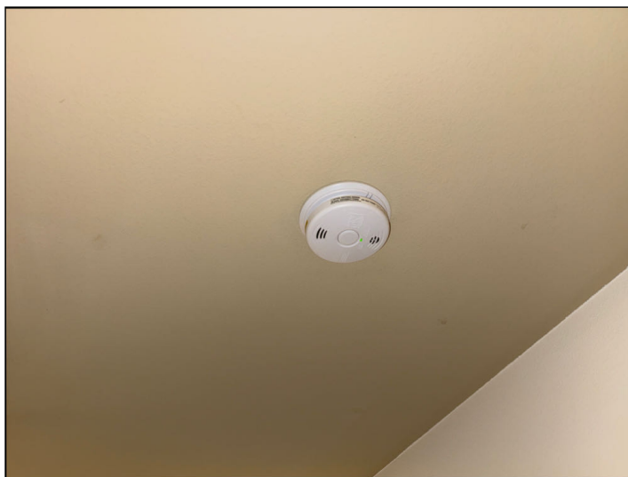
Smoke and CO detectors noted on each floor and inside bedrooms.
