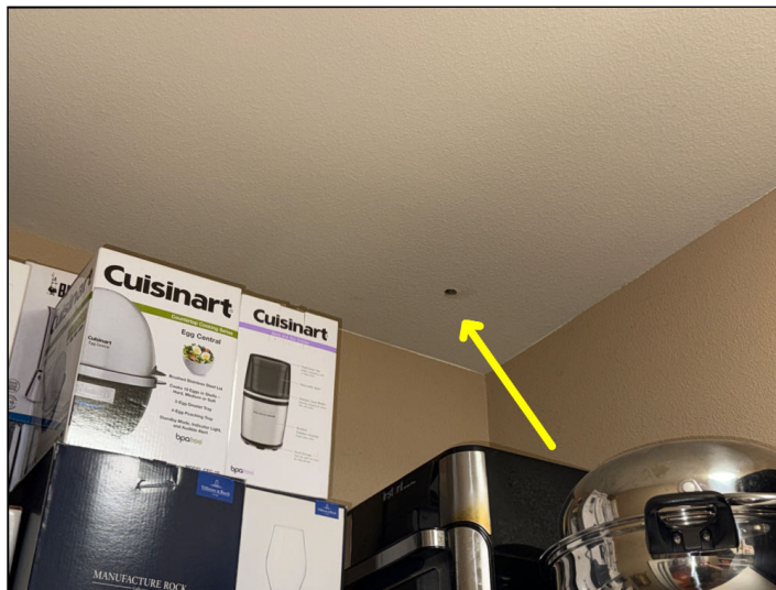
Small hole noted in the pantry ceiling.
