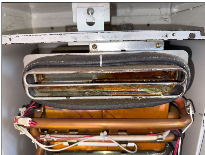
Some corrosion noted at both water heaters vent pipe which is an indication of age.
