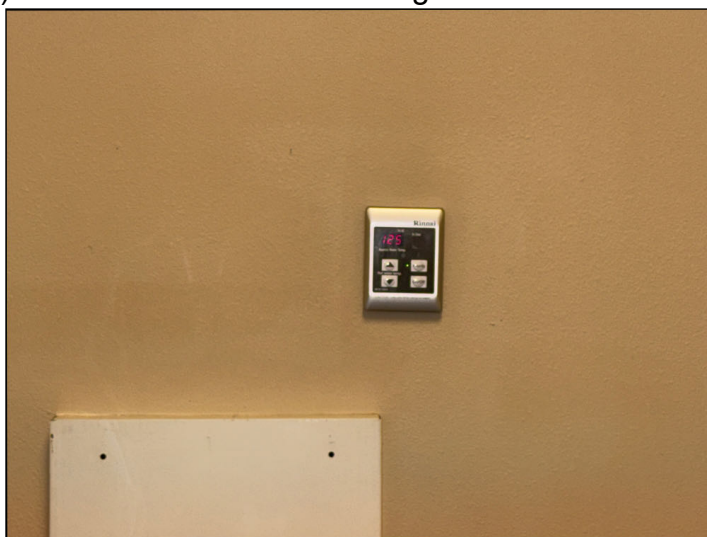
The north water heater temperature is set at 125 which is slightly above the recommended 120.
