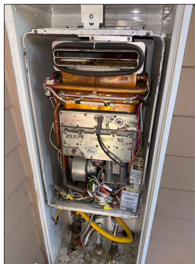
The water heater enclosure is functional.
